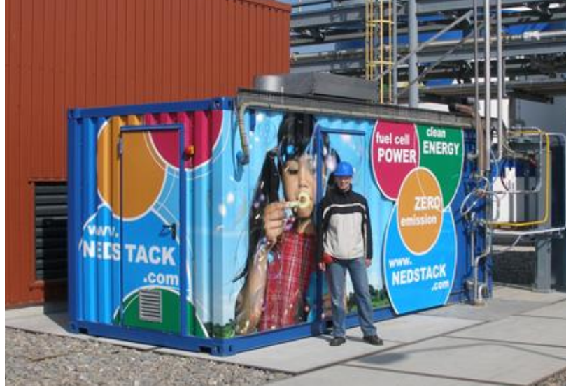
Figure 6.13, Pilot 70 kW PEM fuel cells in container at the Akzo Nobel Chlor-alkali plant in Delfzijl, Netherlands.
