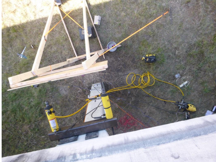
Figure 5-8 Hydraulic Cylinders and Pump Seen From Bridge Deck
