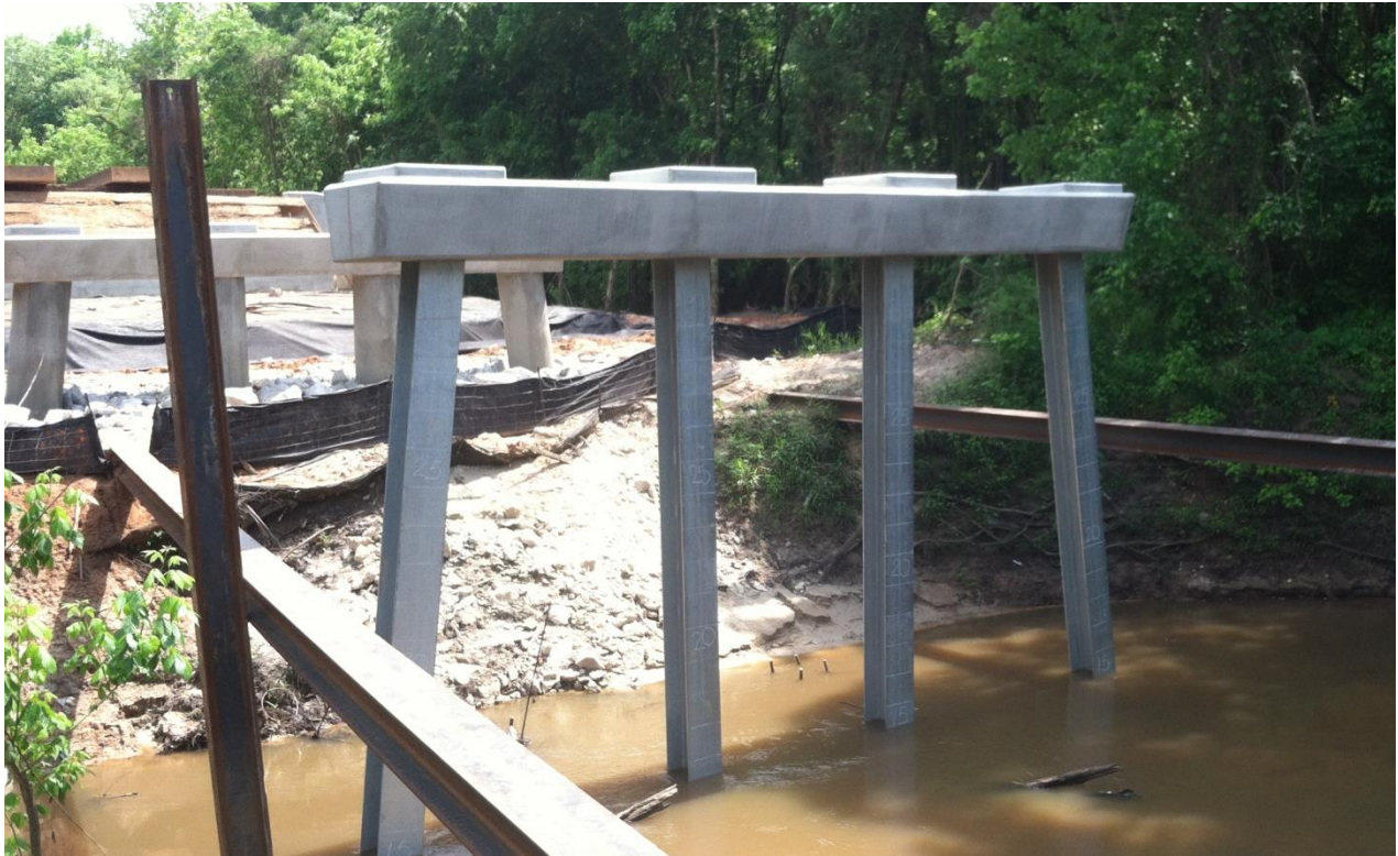
Figure 2-1 Typical Pile Bent with Galvanized Steel HP Piles and Reinforced Concrete Cap
