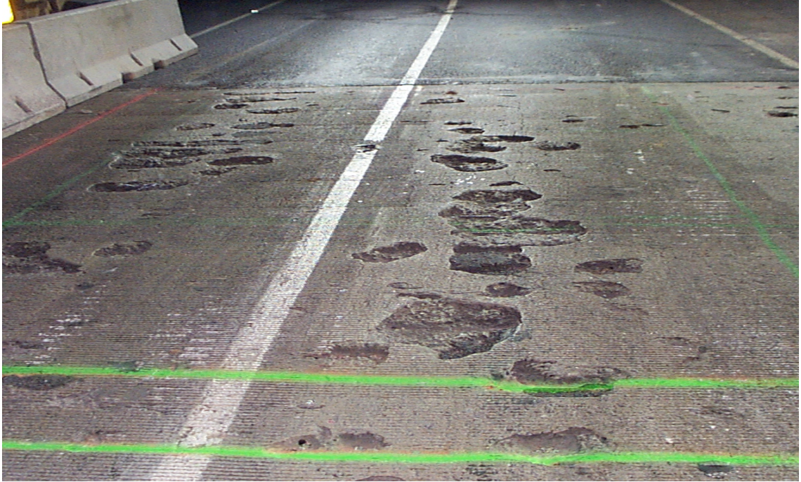
Fig. 5.2 Approach View of Typical Spalling of Original Travel Lanes
