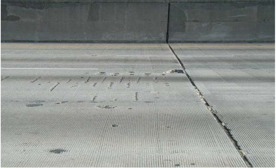
Fig. 2.21 Typical Spalling of Original Lanes (2)
