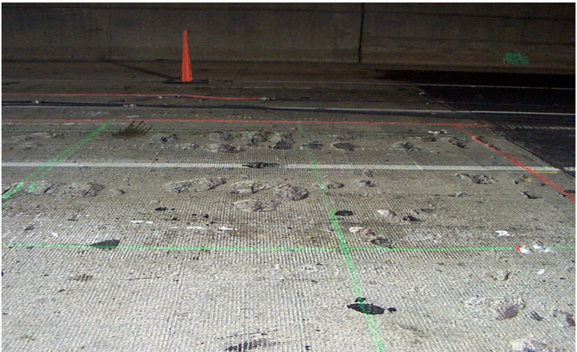
Fig. 5.3 Side View of Spalling of Original Travel Lanes
