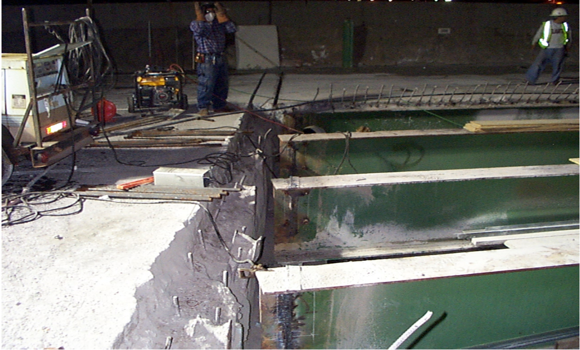
Fig. 6.8 Close-Up of Transverse Edge Beam After the Removal of the Existing Concrete
