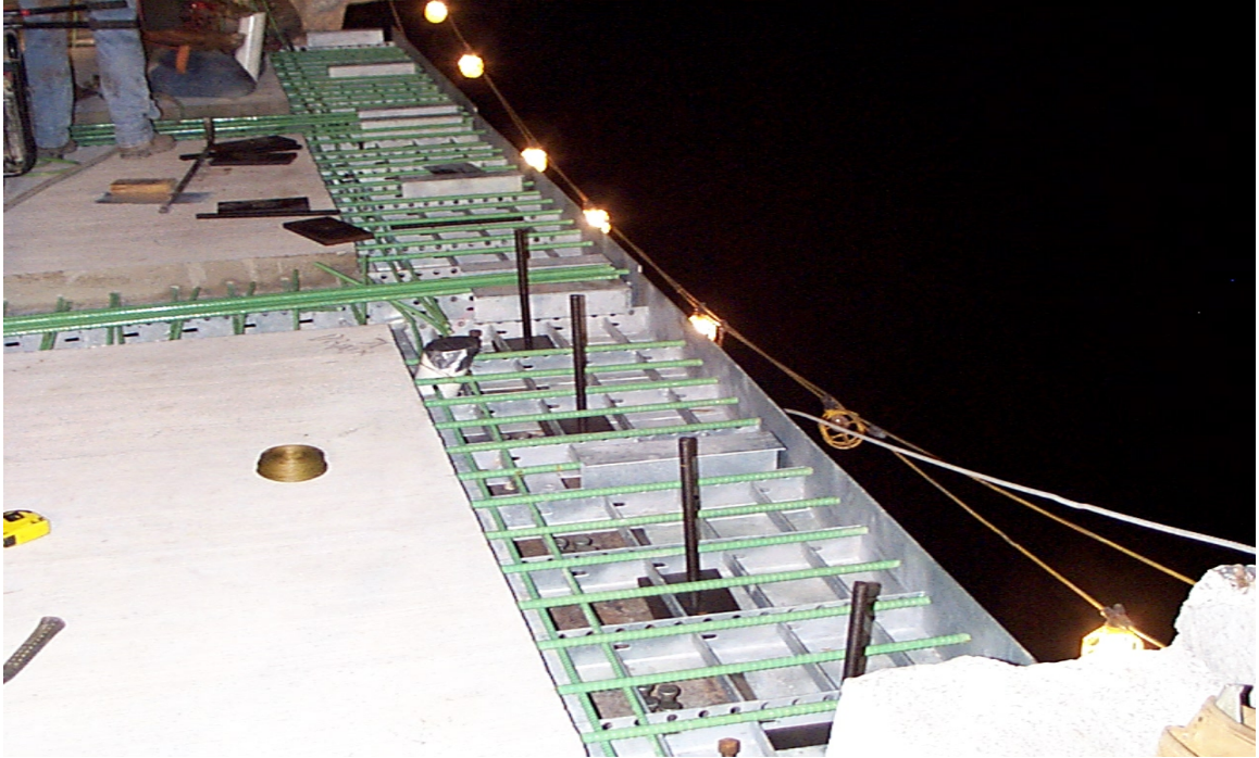
Fig. 4.16 Installation of the Barrier Plates and Bolts for Later Placement of Precast Jersey Barrier Rails
