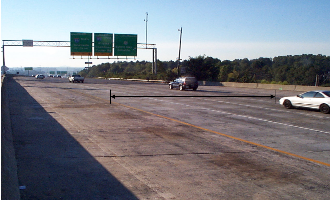
Fig. 6.41 Finished Deck Surface after Deck Replacement Work (between arrowheads) on Eastbound Bridge
