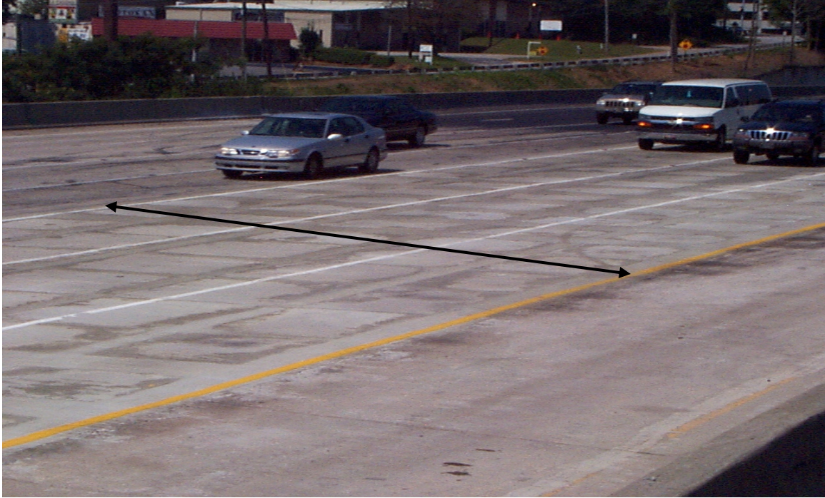
Fig. 6.42 Close-Up of Finished Deck Surface after Deck Replacement Work (between arrowheads) on Eastbound Bridge
