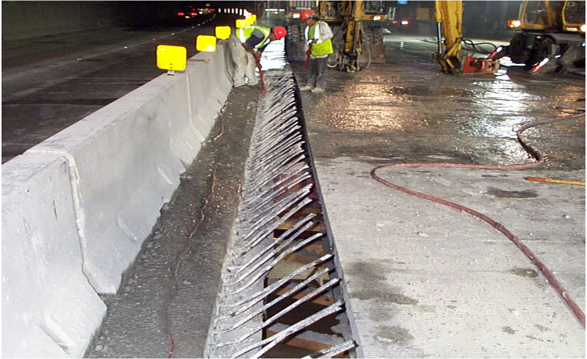
Fig. 5.14 Rebar with Approximately 60° of Bend
