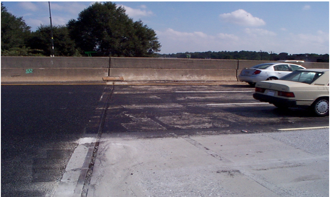
Fig. 7.13 Smearing of Newly Placed Asphalt Wearing Surface Onto New Deck Surface
