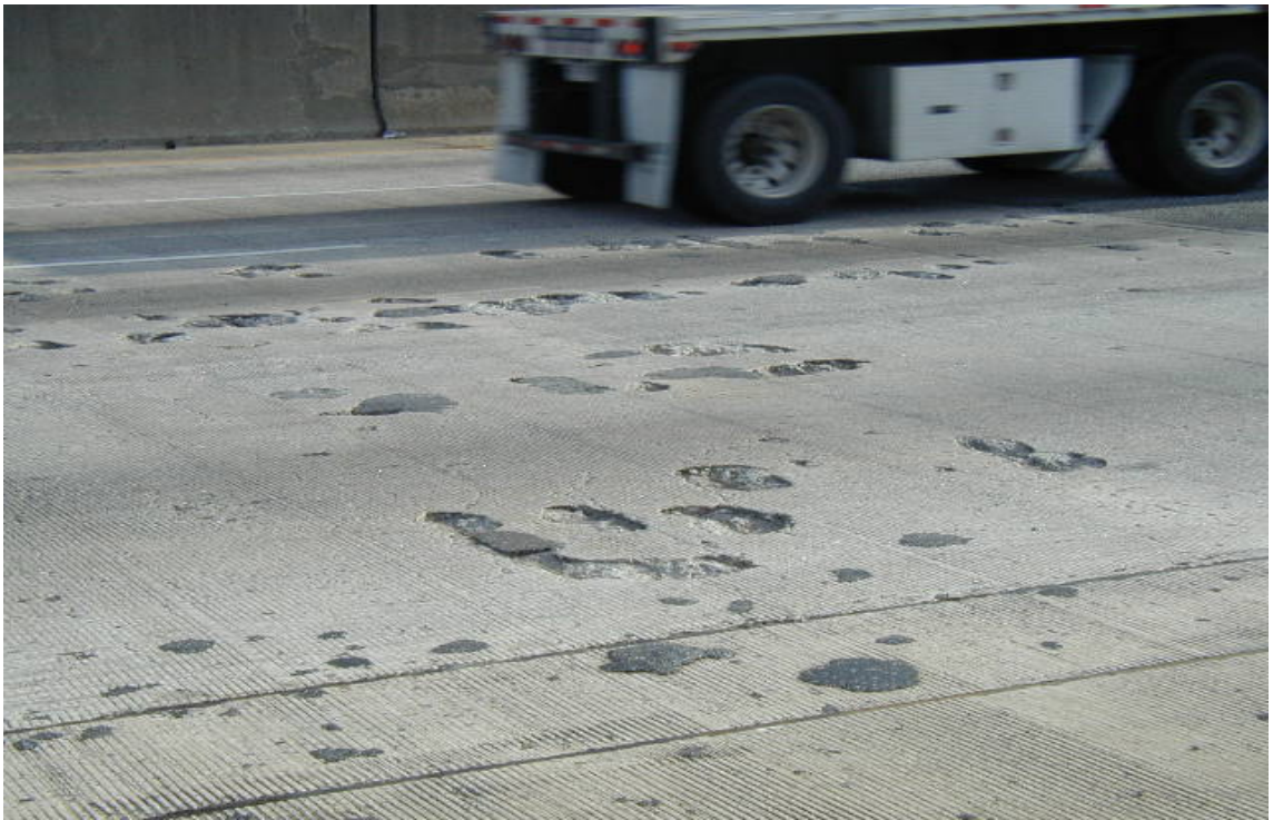
Fig. 2.22 Typical Deck Spalling of Lanes to be Replaced on Northbound Bridge (2)
