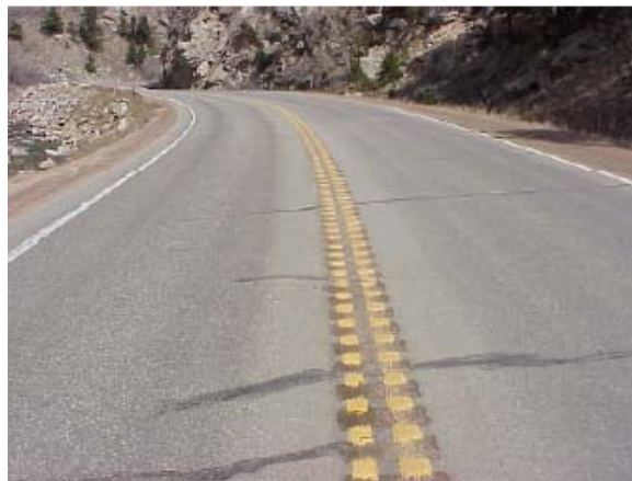
Figure 2.2 Centerline Rumble Strips on State Highway 119 in Boulder Canyon, Colorado, (Report CDOT-DTD-R-2001-8).
