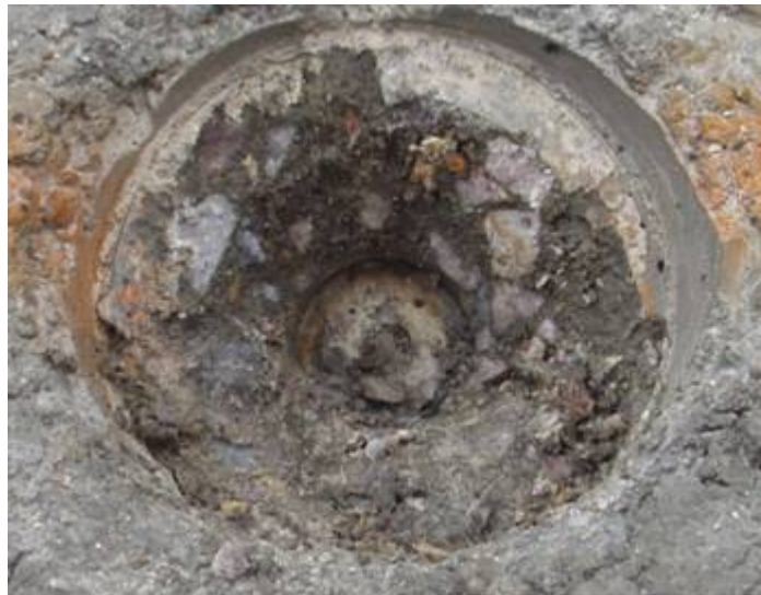
Figure B-91: Top pullout insert completely removed
