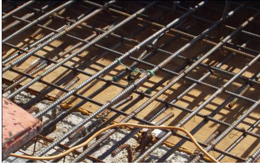
Figure C-121: iButtons on overhang of the Creek Bridge
