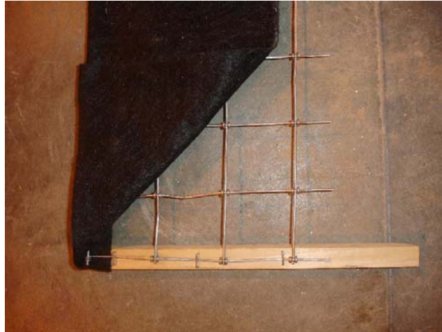
Figure 4.25 Small-Scale Type A Silt Fence.
