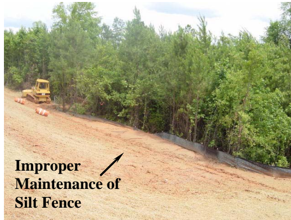
Figure 3.4 Failure Mode: Improper Maintenance.
