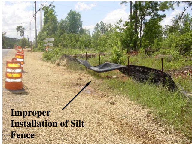
Figure 3.5 Failure Mode: Improper Installation.
