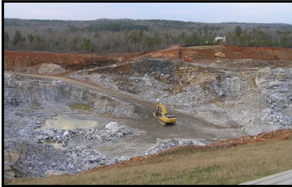
Figure 2. Photograph (taken Fall 2009) of the quarry site looking east from the west highwall.
