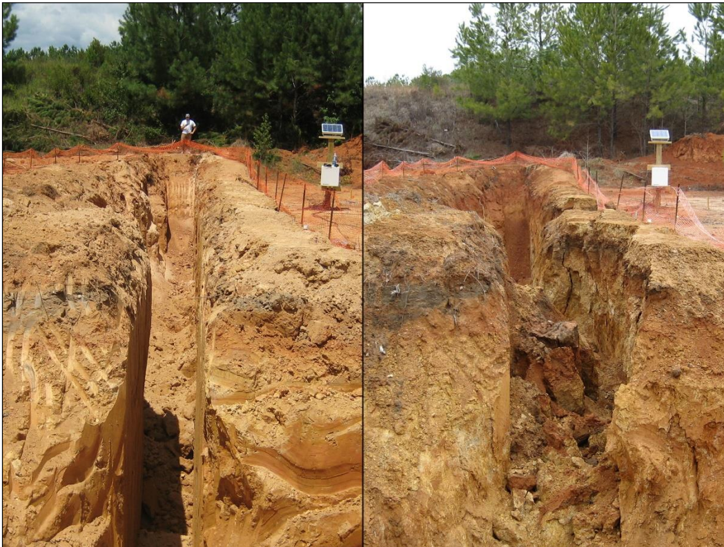
Figure 56 - Excavation #1 before and after failure (North facing).
