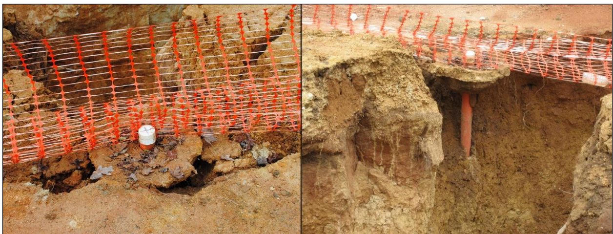
Figure 71 - Inclinometer casings after failure (Excavation #1).
