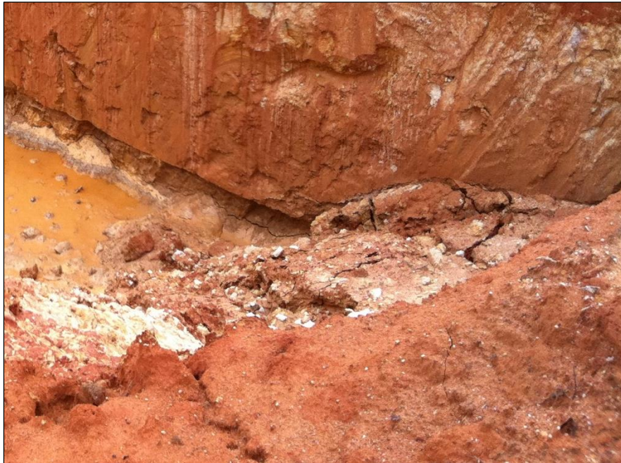
Figure 53 - Undermining from water in bottom of trench.
