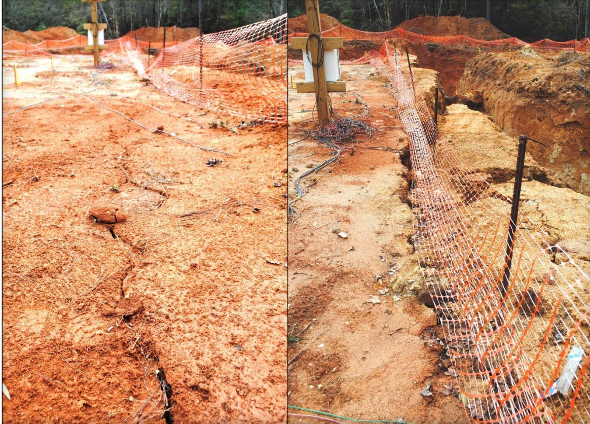
Figure 62 - Tension crack progression over time (Excavation #1).
