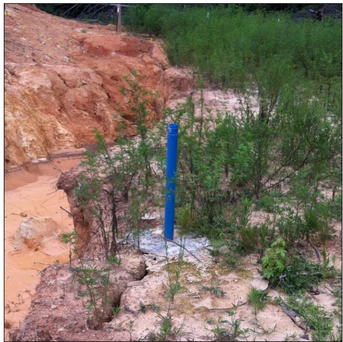
Figure 73 – Inclinometer casing after failure (Excavation #2).
