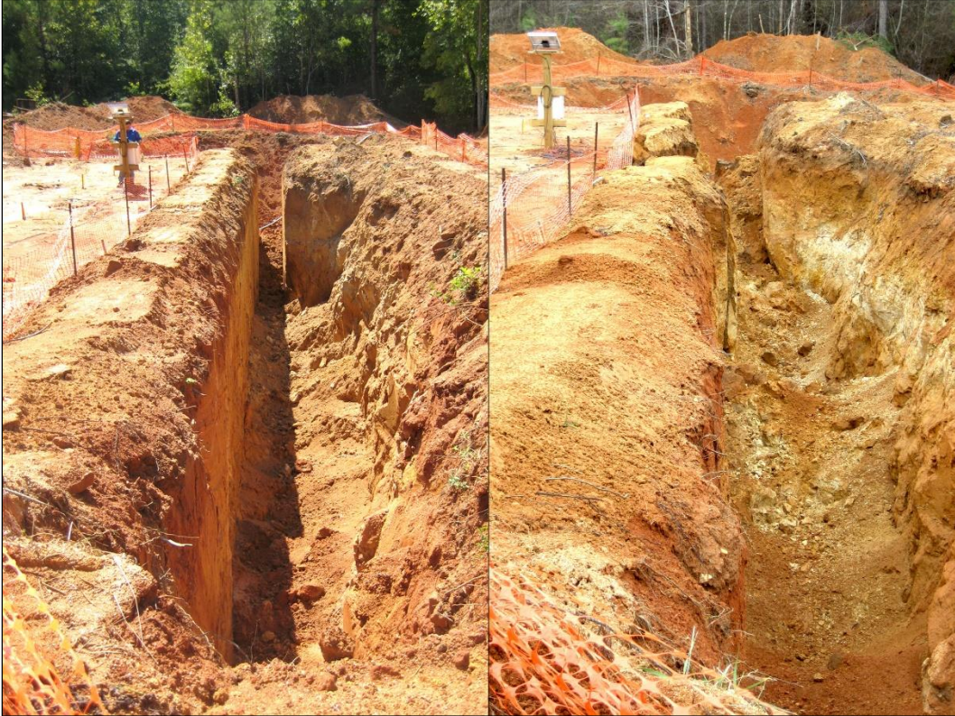
Figure 55 - Excavation #1 before and after failure (South facing).
