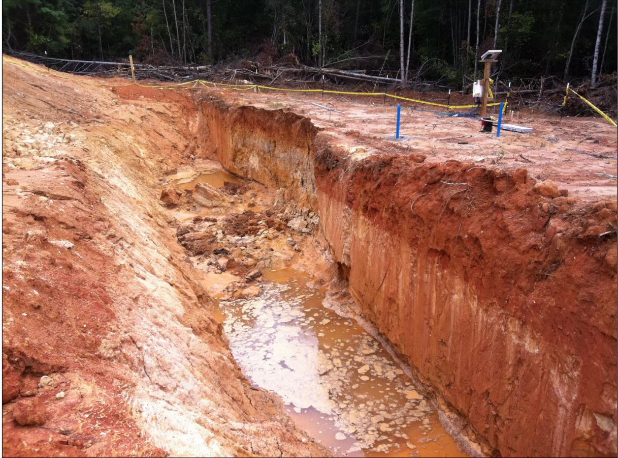
Figure 59 – Excavation #2 after initial failure on 9/21/11.
