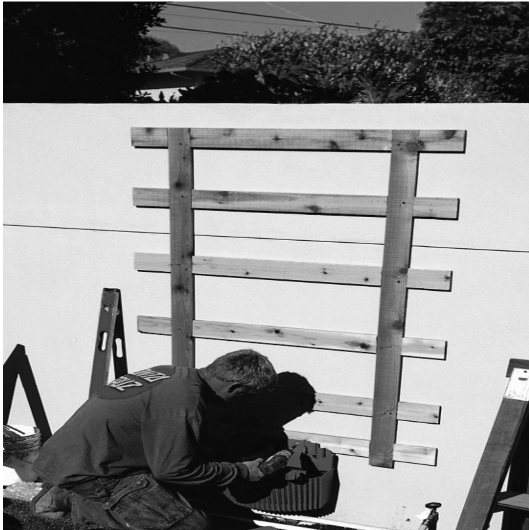
Figure 4.16. Prior to attaching the living wall planters for the Woolly Pocket living wall design shown in Figure 15, a wooden structural support system was installed onto a concrete wall.
