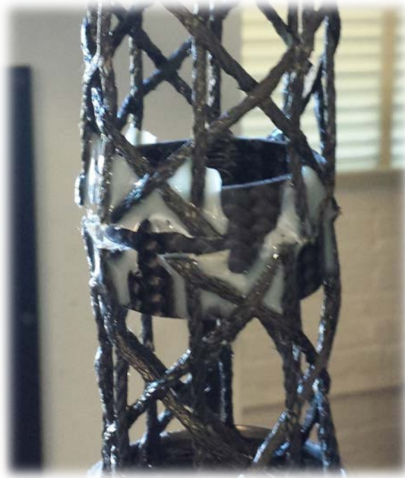
Figure 65 – Failure of 1 inch Splice Joint
