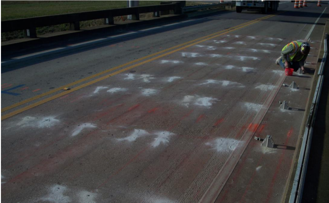
Figure 4.20 Anchors in the Bridge Deck for Saw Track
