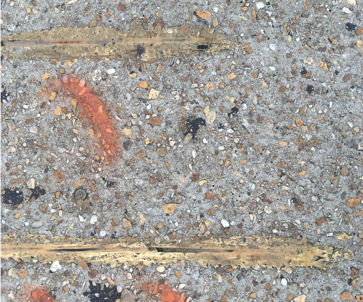
Figure 6.18 Degradation of Epoxy Near Ends of Strips
