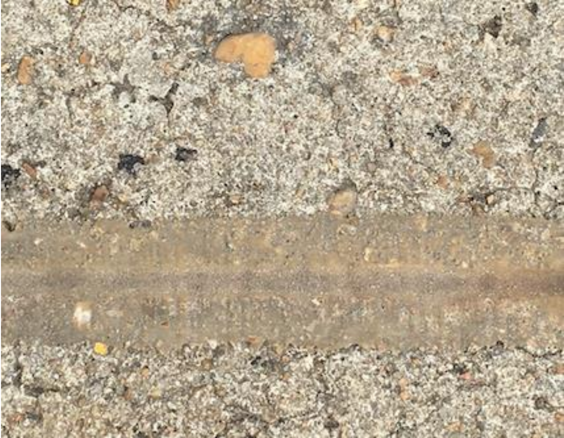
Figure 6.16 Epoxy Showing No Degradation One Year After Installation
