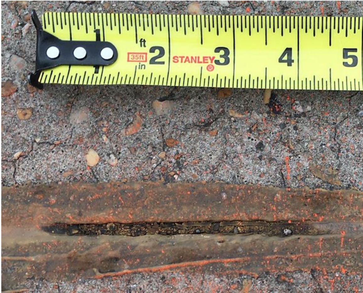
Figure 6.17 Typical Area of Epoxy Degradation
