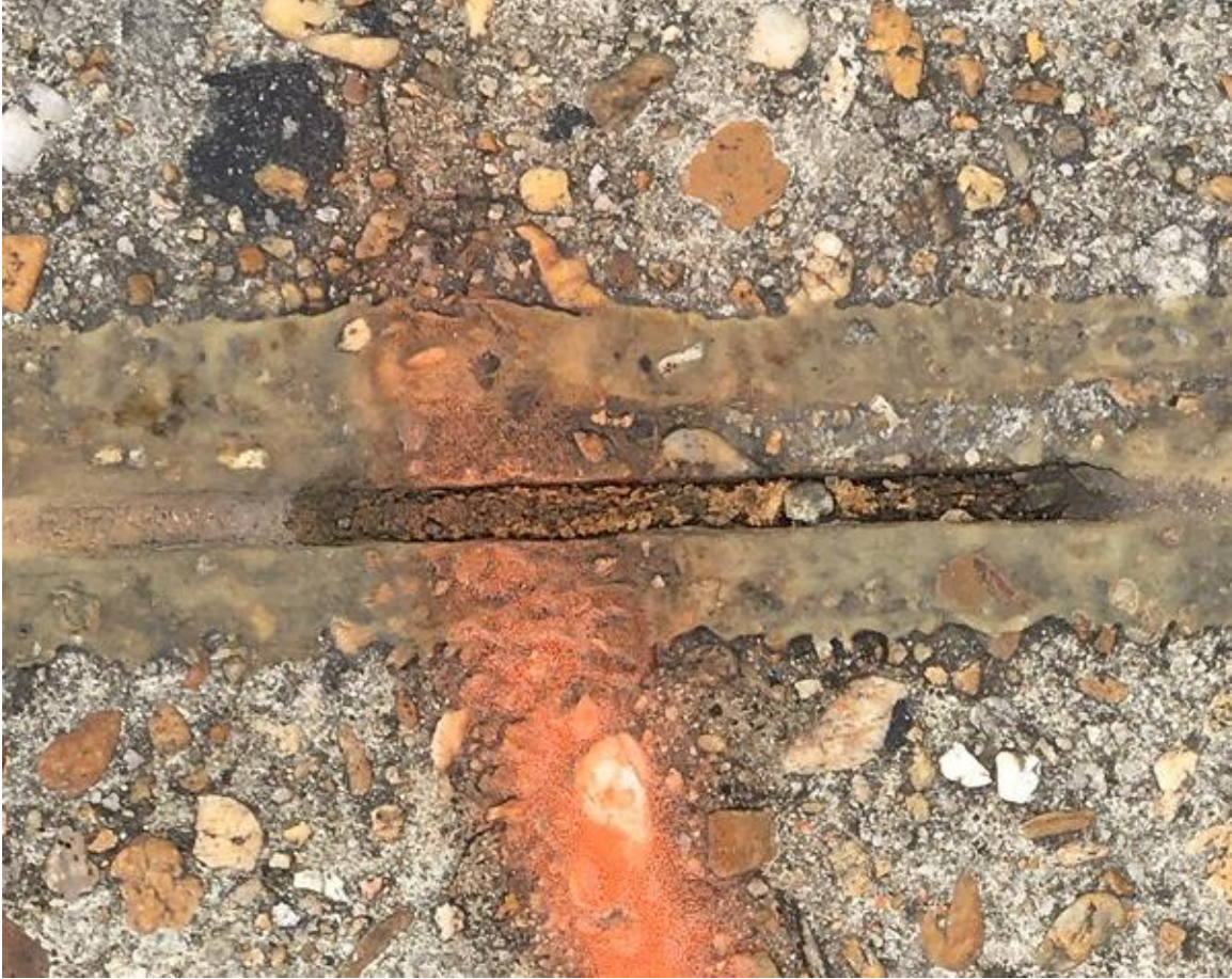
Figure 6.19 Typical Epoxy Degradation
