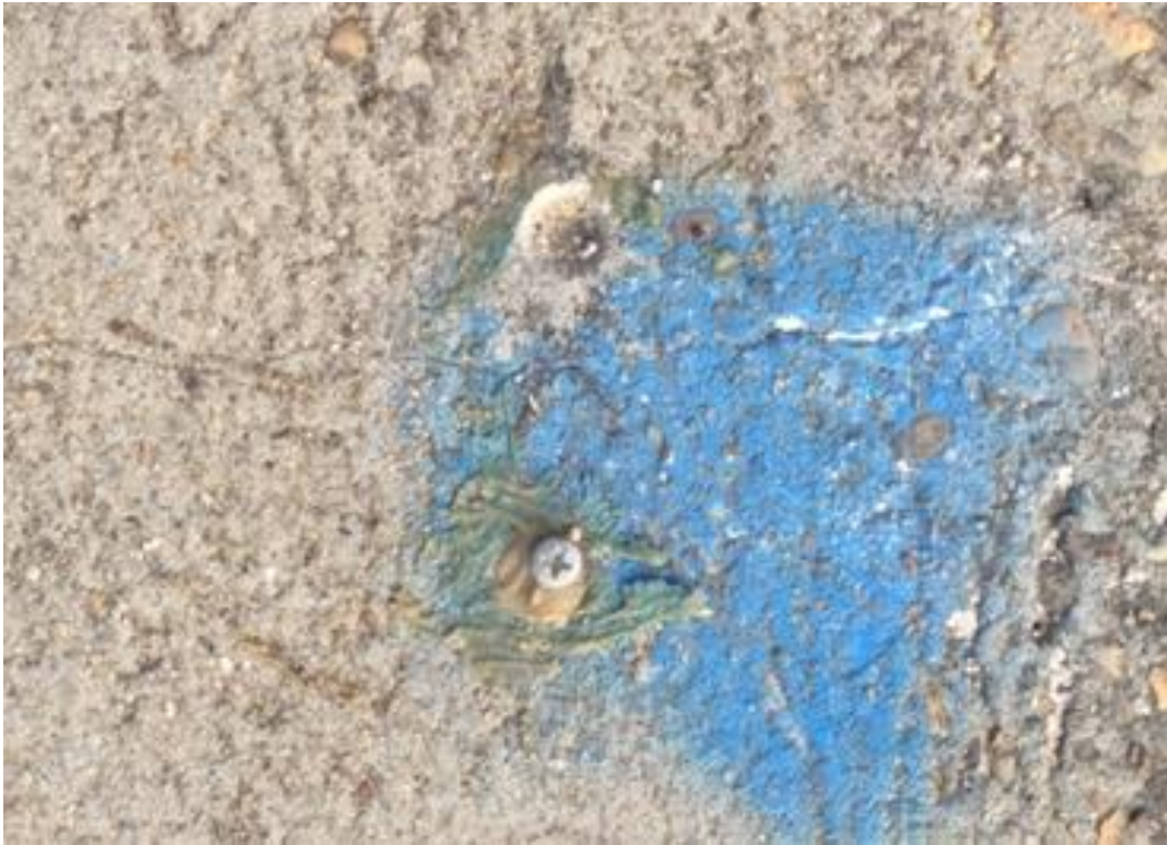
Figure 5.22 Transducer Mount Damaged by Traffic
