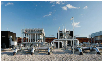
Figure 15. Hilabee Power Plant view. Alex city.
