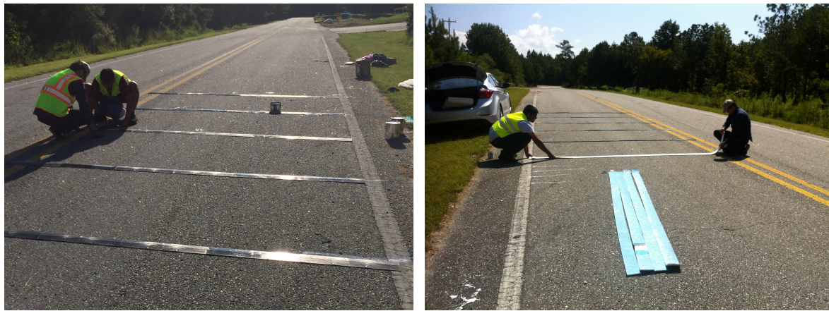
(a) (b) Figure 8 DRS Installation (a: TAPCO; b: ATM)
