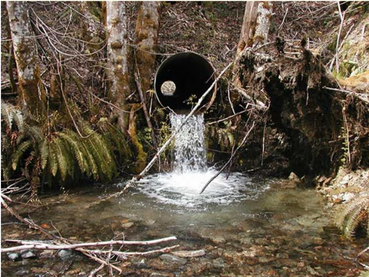
Figure 2-39: Culvert Barrier to Fish Passageway (USDA 2005)
