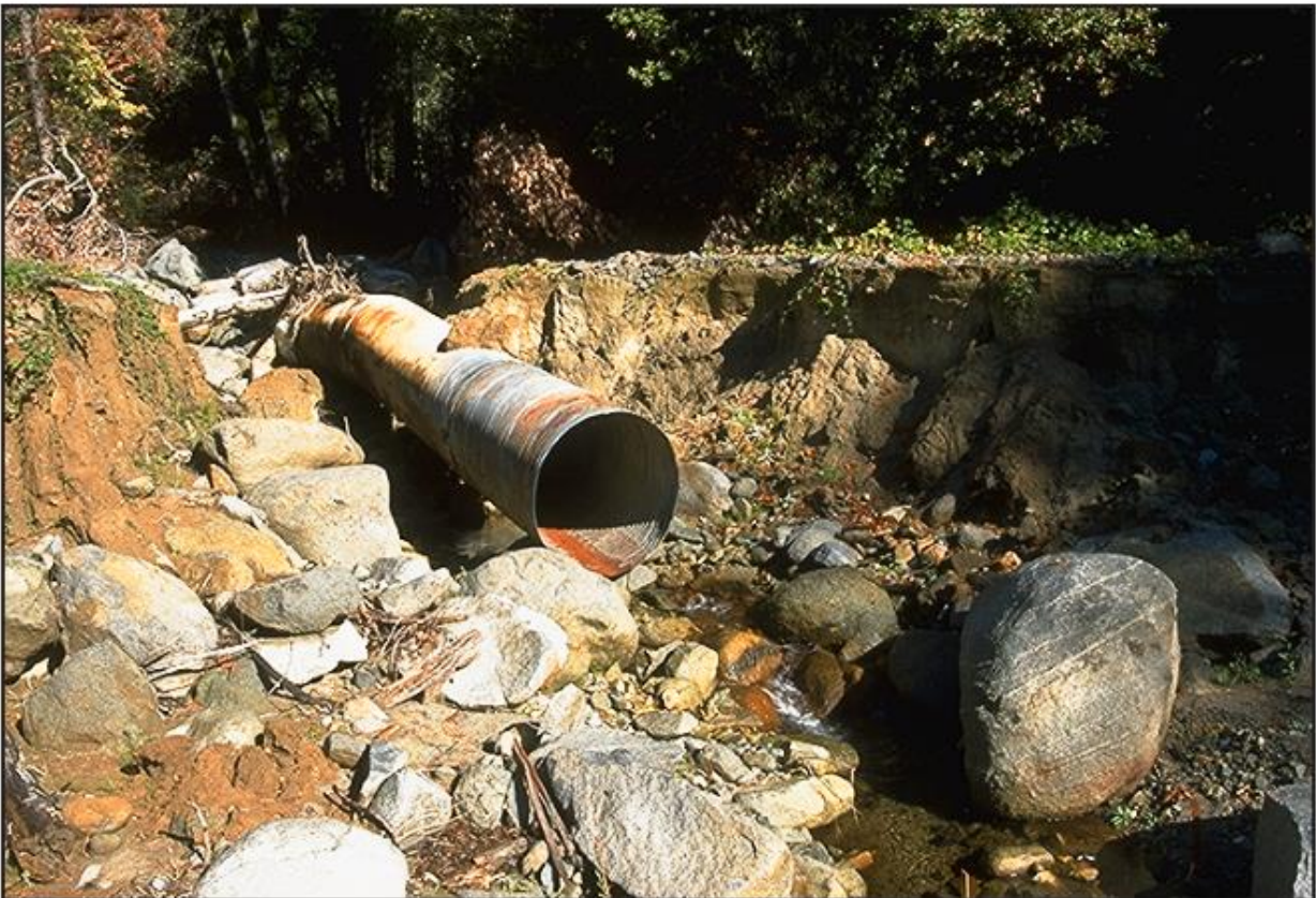
Figure 2-42: Inadequately Designed Culvert (Keller 2003)
