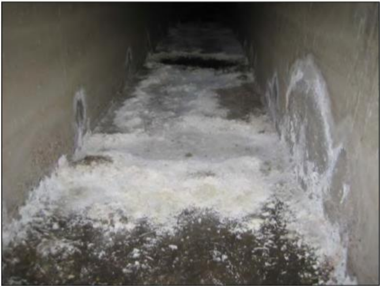
Figure 2-21: Corrosion of Reinforced Concrete Culvert (Molinas 2009)
