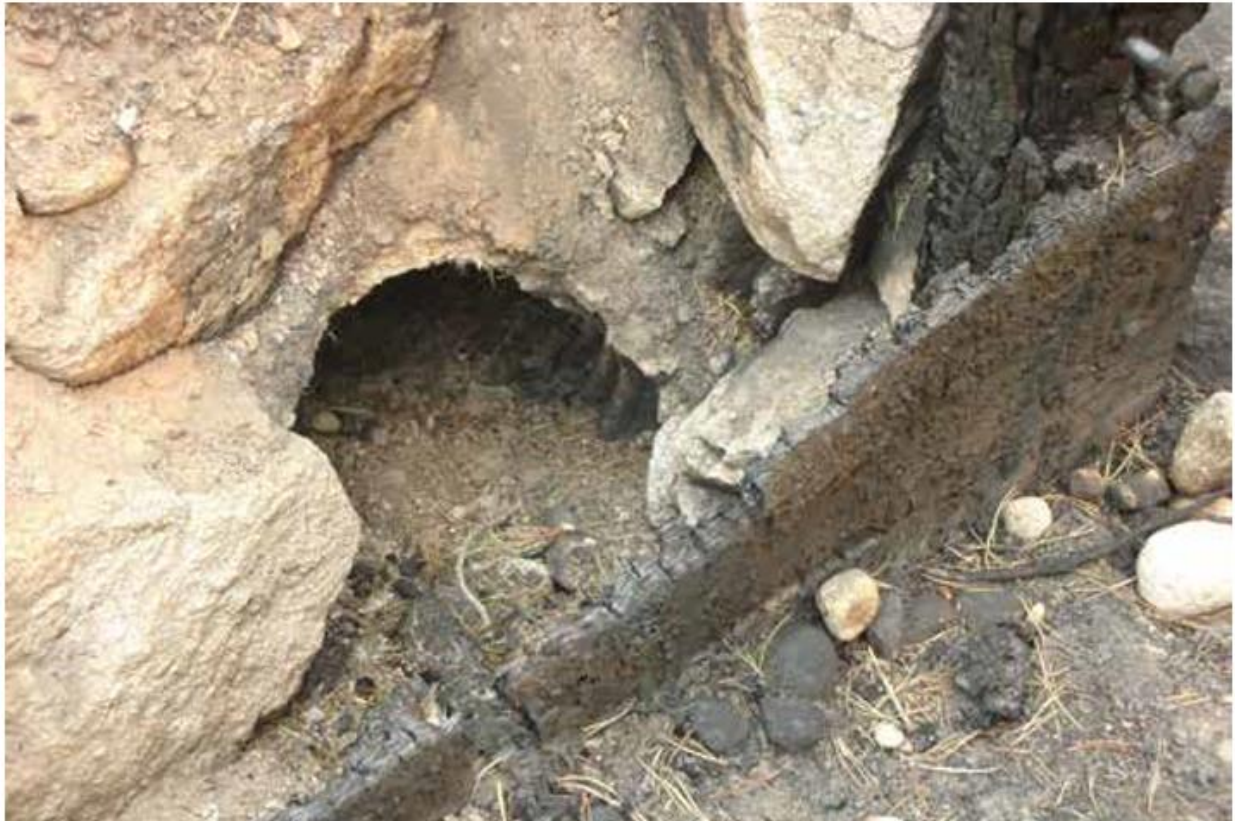
Figure 2-34: Burned High Density Polyethylene Inlet (Kestler 2012)
