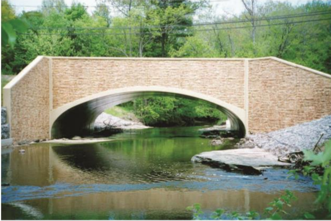
Figure 2-40: Bottomless Culvert for Aquatic Organism Passage (GDOT 2014)
