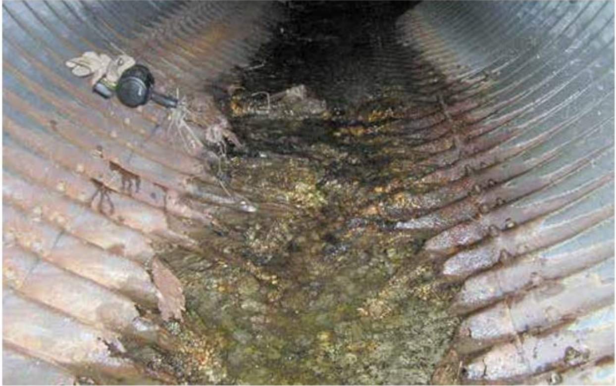
Figure 2-22: Corrosion of Corrugated Metal Culvert (Kestler 2012)
