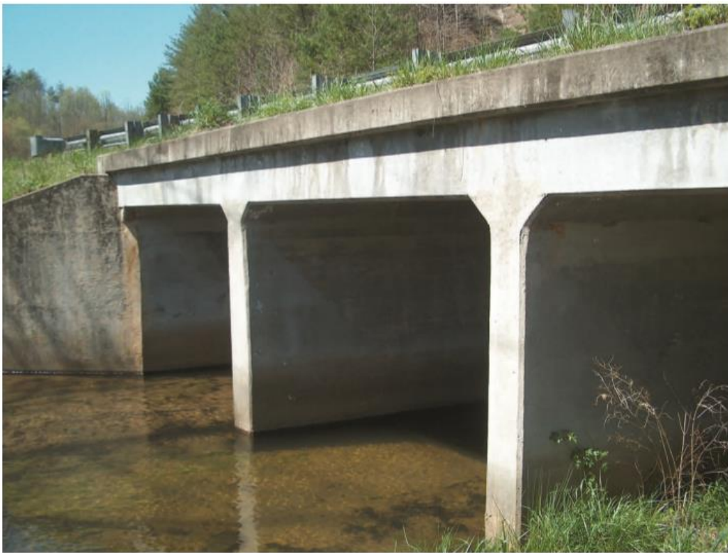
Figure 2-41: Embedded Box Culvert for Aquatic Organism Passage (GDOT 2014)
