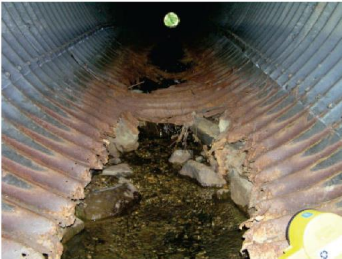
Figure 2-28: Corrosion Accelerated by Abrasion of Metal Culvert (NCHRP 2015)
