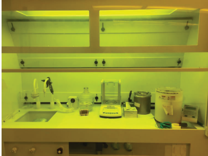
Figure 4.3-2: Picture of one of cleaning fume hood in Physics' Departments clean room facilities.
