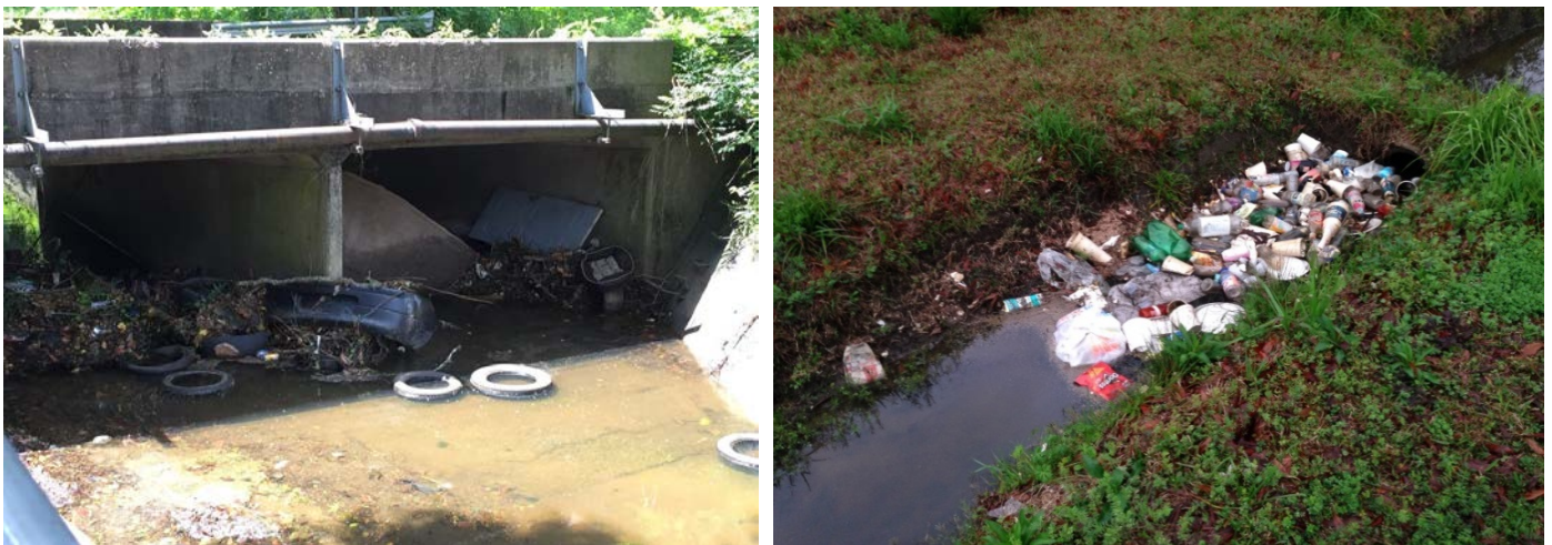
Figure 3. 24. The channel being clogged by vegetation and trash at site 5
