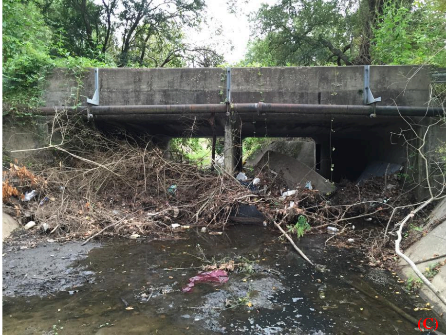
Figure 2.6: Water backed up due to the channel being clogged below the West Prichard Avenue Bridge
