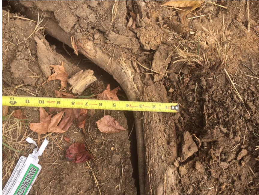
Figure 111: Tree Root (4" Diameter) Approximately 15' from Edge of Pavement
