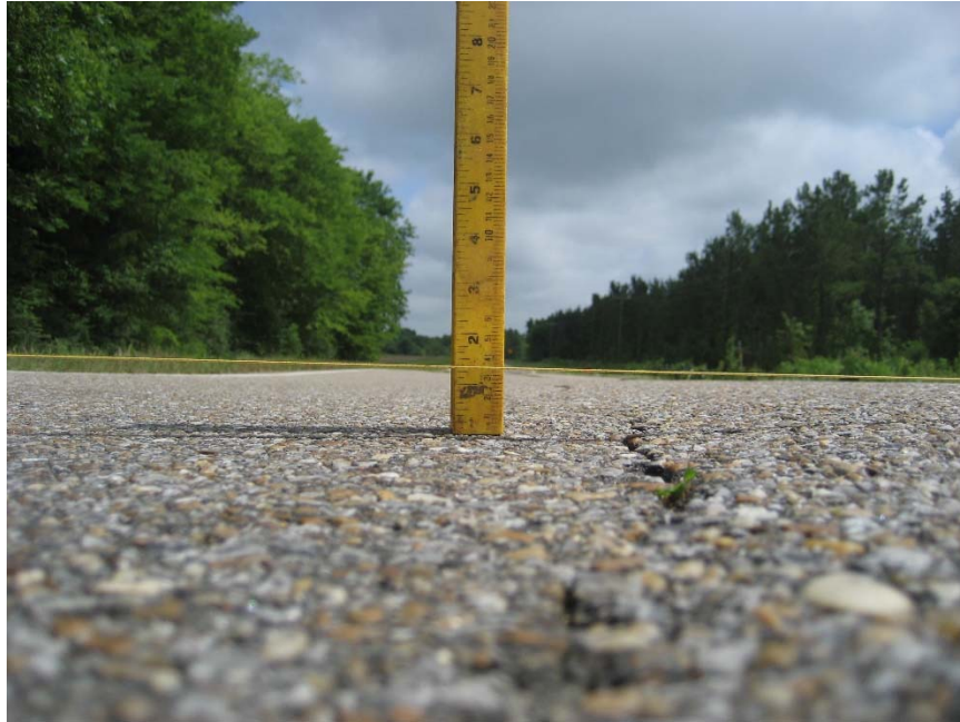
Figure 84: Observed Rutting Near Boring 5.0 MP 52.85 (Rut Depth 1 \frac{3}{8} inch)
