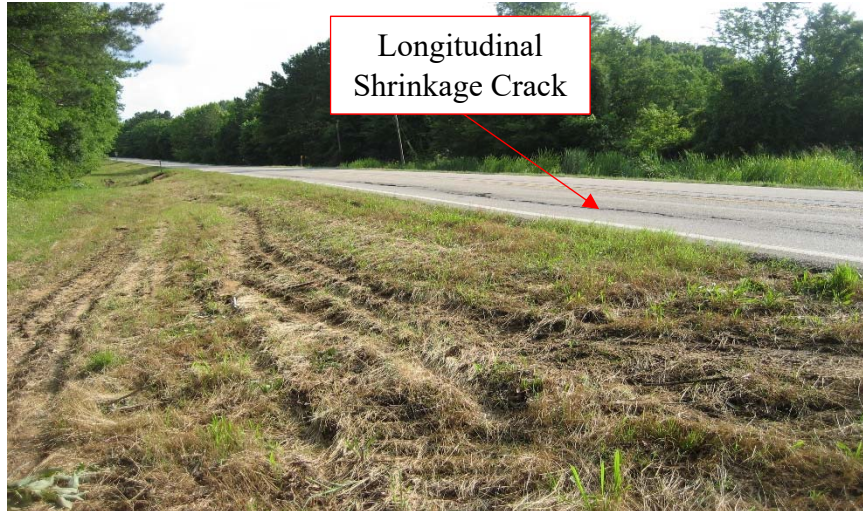
Figure 81: Longitudinal Crack due to Shrink Swell near Boring 5.0 MP 52.85 (Photo Taken 06/02/15)
