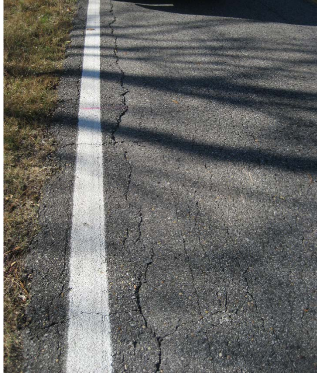
Figure 36: Longitudinal Edge Crack at AL-5
