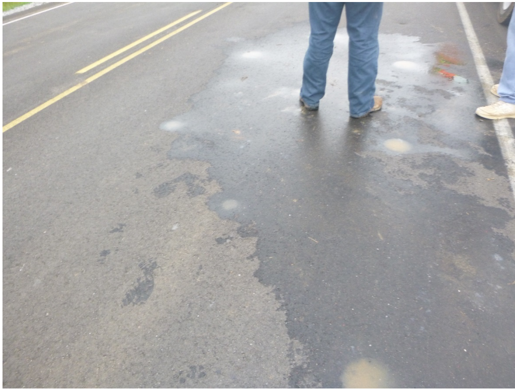
Figure 34: Lime Columns Reflected Through Binder Course and Holding Water
