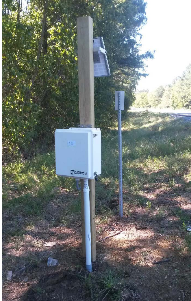
Figure 59: Data Acquisition Installation
