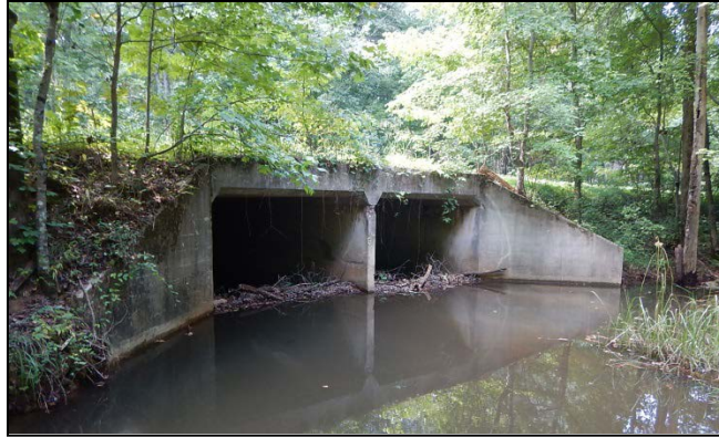
Plate 5: Culvert backup at a road-cut in Osborn Creek.
