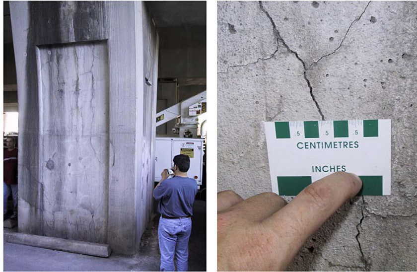
Figure 2-11: Cracking Due to DEF at San Antonio Y Overpass (Thomas et al., 2008)
