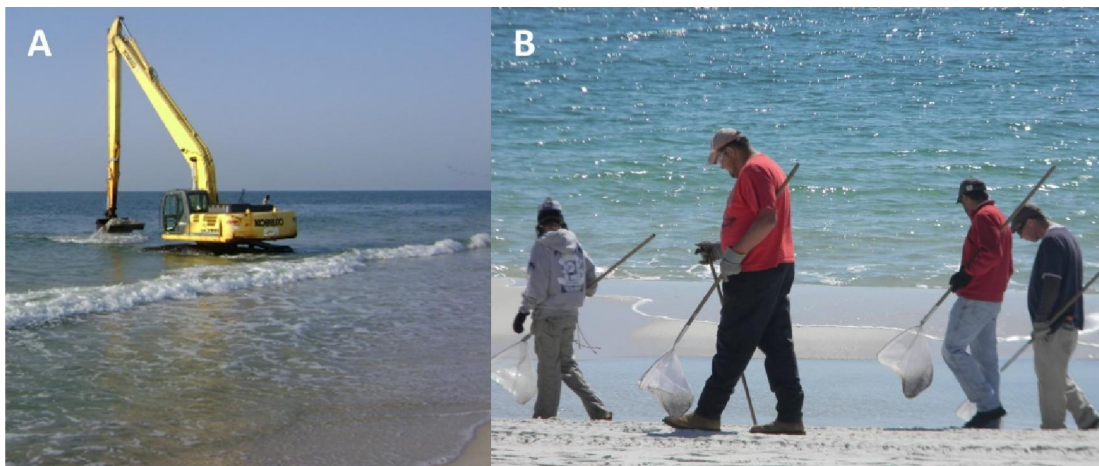
Figure 2-11. A) An excavator removes a submerged oil mat that resulted from the Deepwater Horizon oil spill. B) A team of volunteers collects SRBs along the shoreline.
