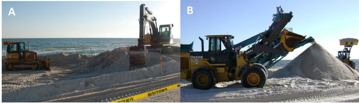
Figure 2-10. Sediment contaminated by SRBs from the Deepwater Horizon oil spill being A) excavated and then B) sifted and returned to the beach.
