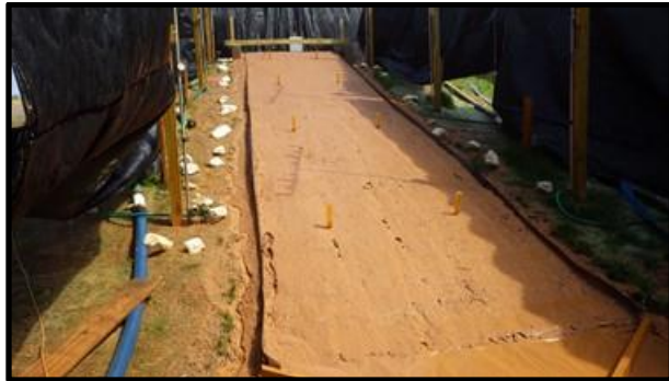
(c) slope erosion after interval 2
