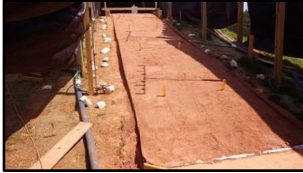
(a) slope conditions before test
