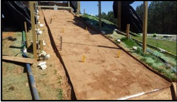
(a) slope conditions before test
