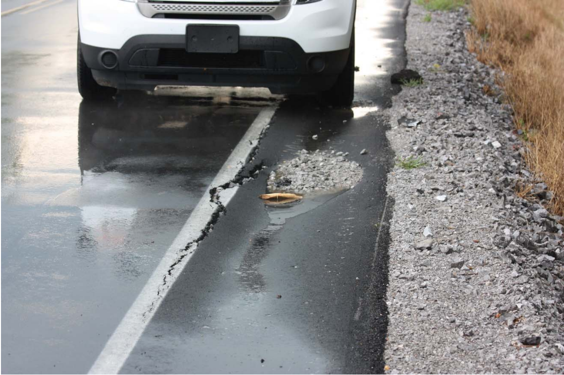
Figure 51: Rutting Observed above Vertical Barriers
