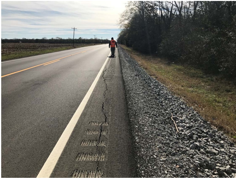
Figure 91: Longitudinal Crack in Vertical Barrier Test Section
