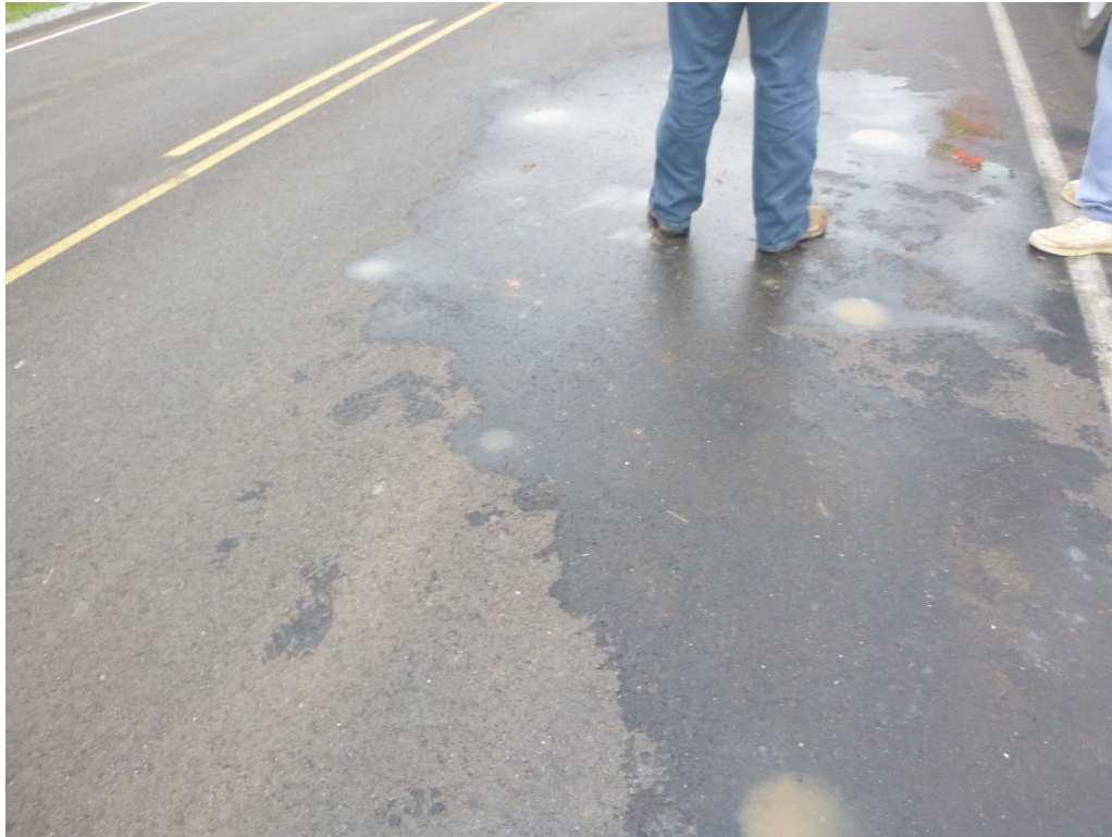
Figure 62: Lime Columns Reflected Through Base Course and Holding Water
