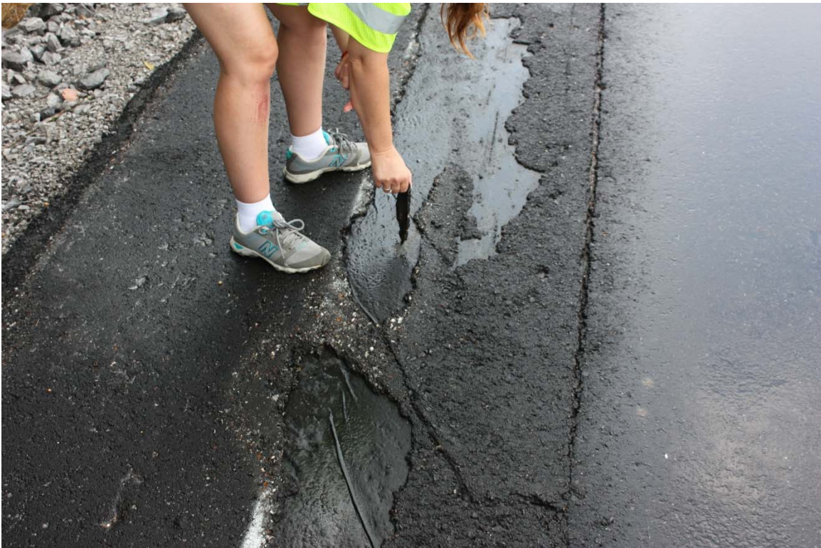
Figure 52: Asphalt Spalling above Vertical Barriers
