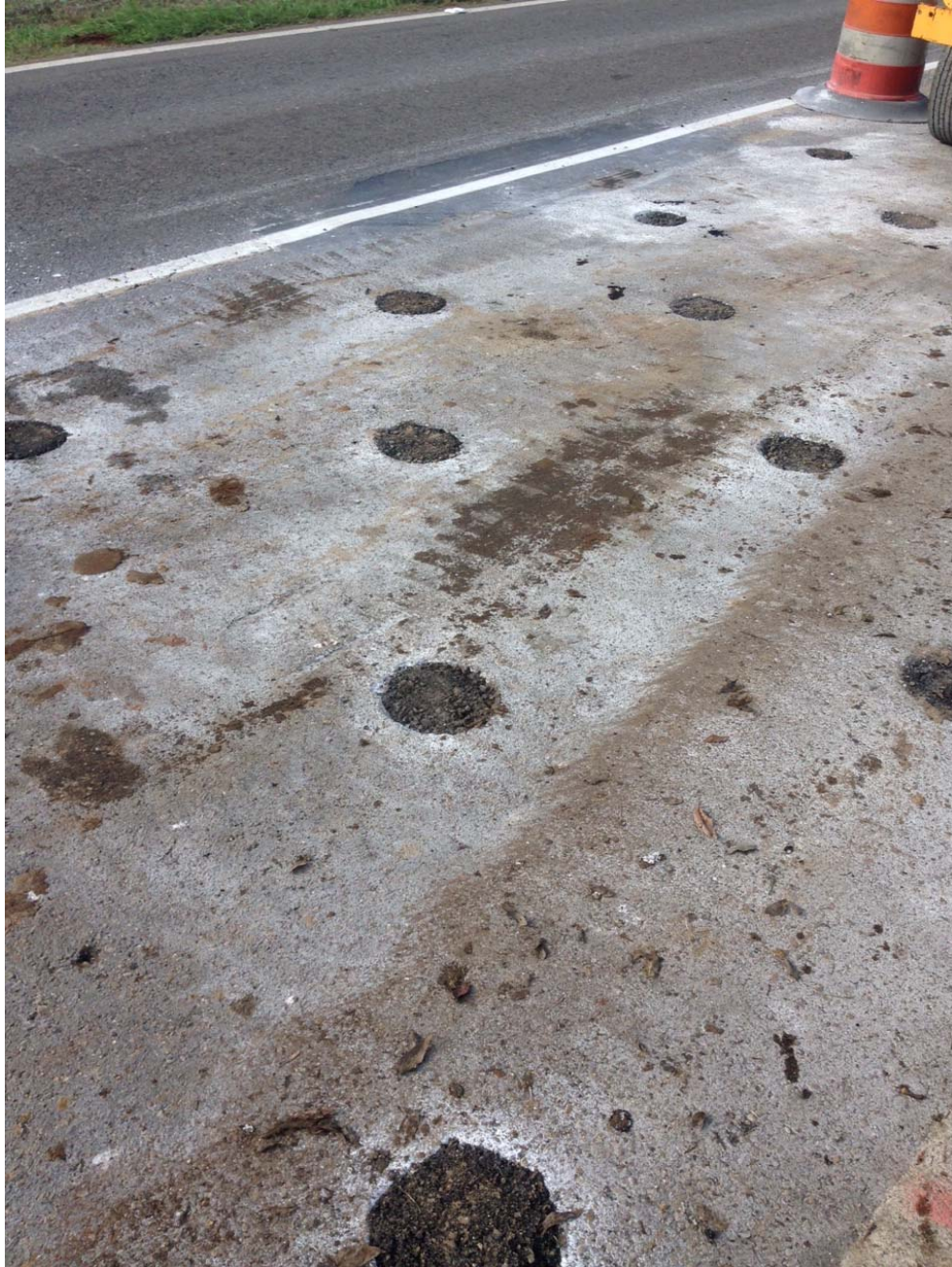
Figure 61: Lime Columns patched with Asphalt
