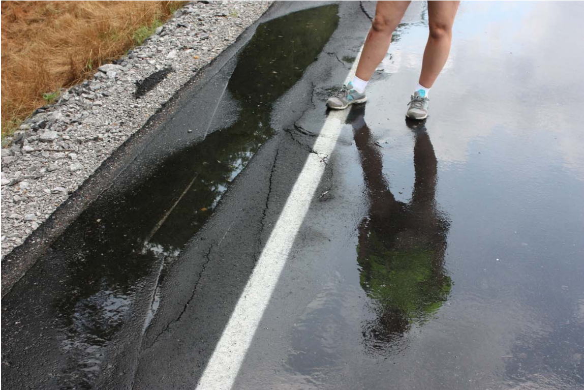
Figure 50: Cracks along shoulder above Vertical Barriers
