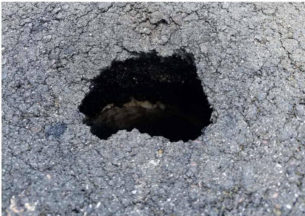
Figure 63: Hole in Asphalt above Lime Column
