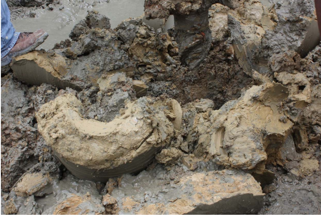
Figure 75: Clumps of soil showing lack of cement mixing
