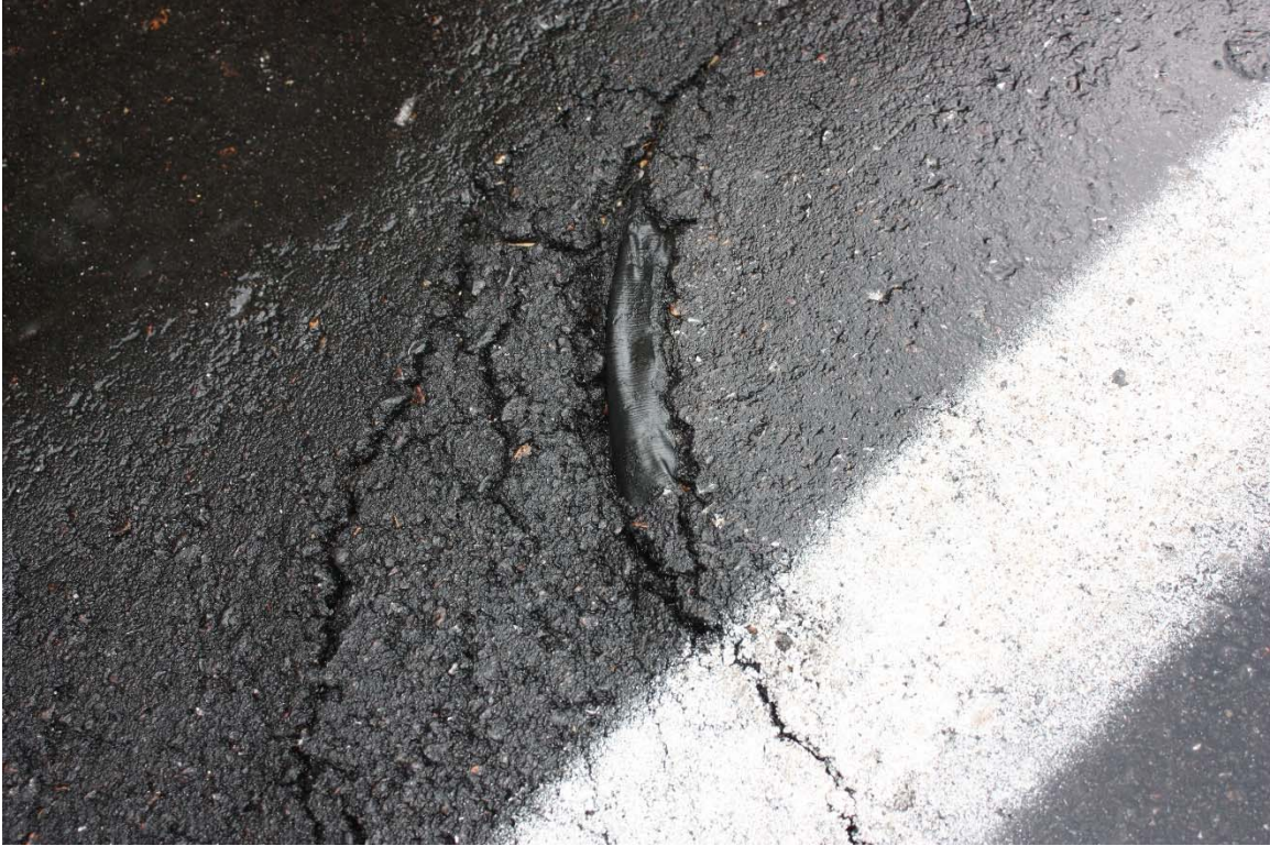
Figure 53: Geosynthetic protruding through base course of asphalt
