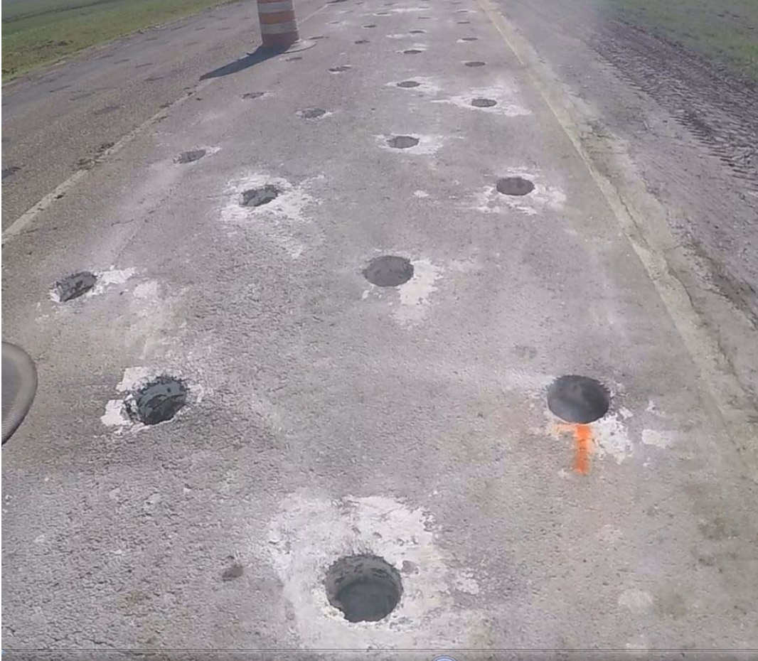
Figure 58: Lime Column before Asphalt Patching
