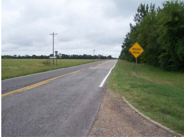
Figure 1: Distresses Pavement at AL-5 (Herman 2015)
