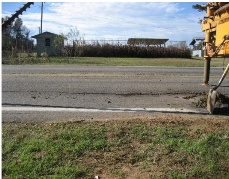
Figure 2: Longitudinal Cracking at AL-5 (Herman 2015)
