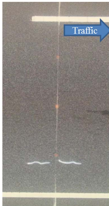
Figure 6.10 – Longitudinal cracking on 2009-S9 RL#3 on 8/19/2013.
