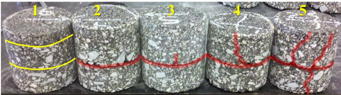
(b) Cores taken from Original High RAP section with cracking and delamination highlighted.
