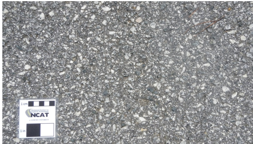
Figure 3.15 - Surface condition of pavement.
