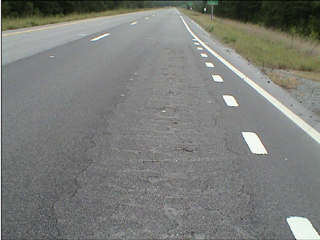
Figure 6.13 – Fatigue cracking in 2003-N1 (Priest and Timm, 2006)
