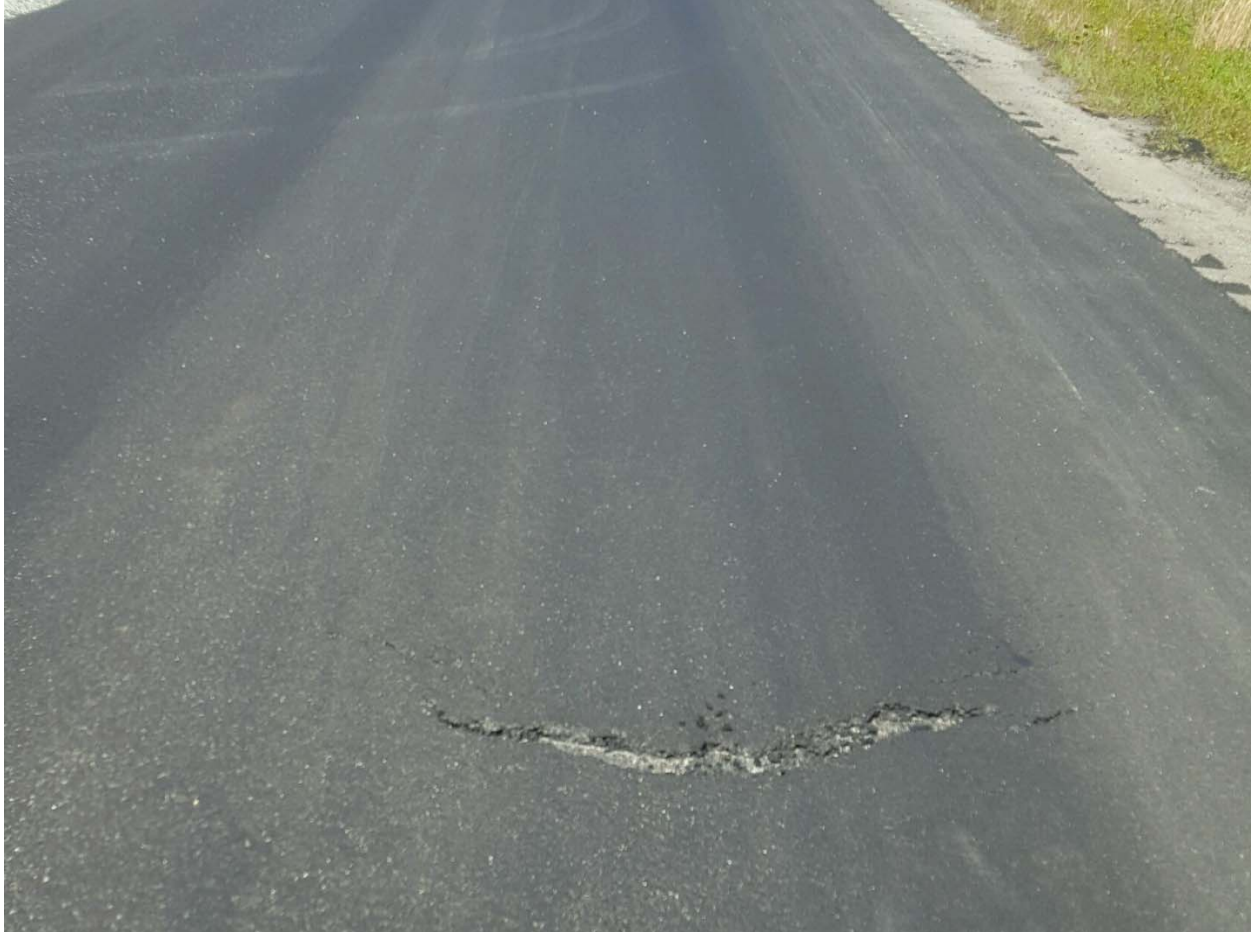
Figure 2.6 – Crescent shaped cracking resulting from delamination of the surface layer.
