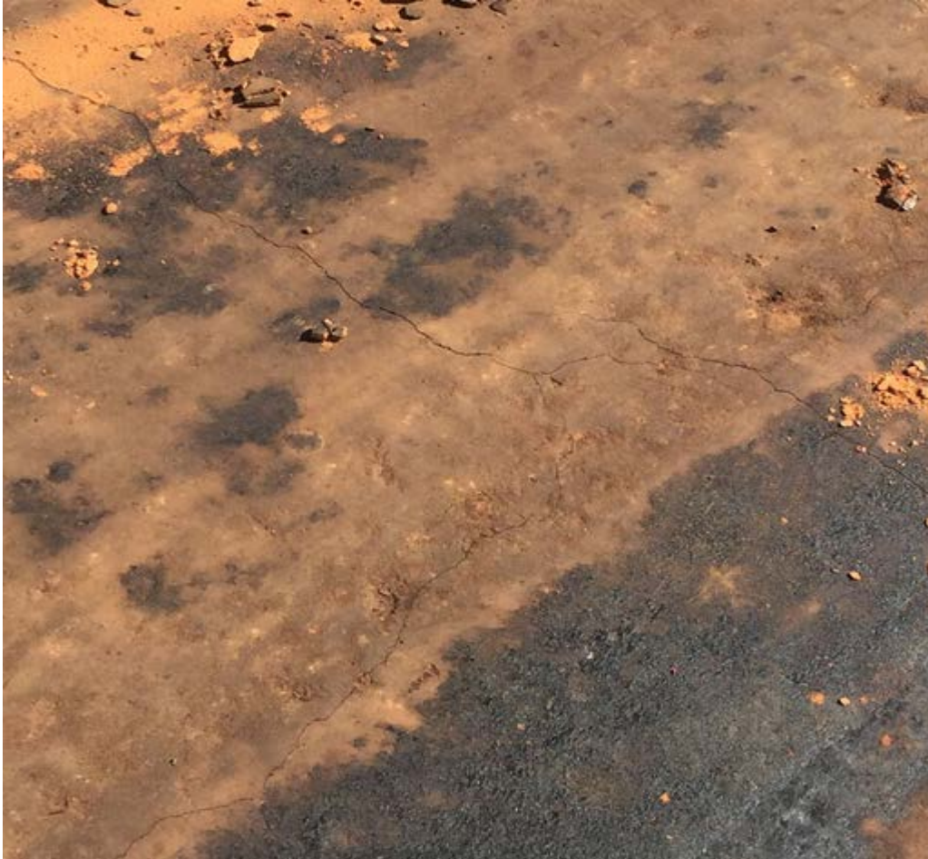
Figure 2.5: Transverse and Longitudinal Cracking on U.S. Highway 84
