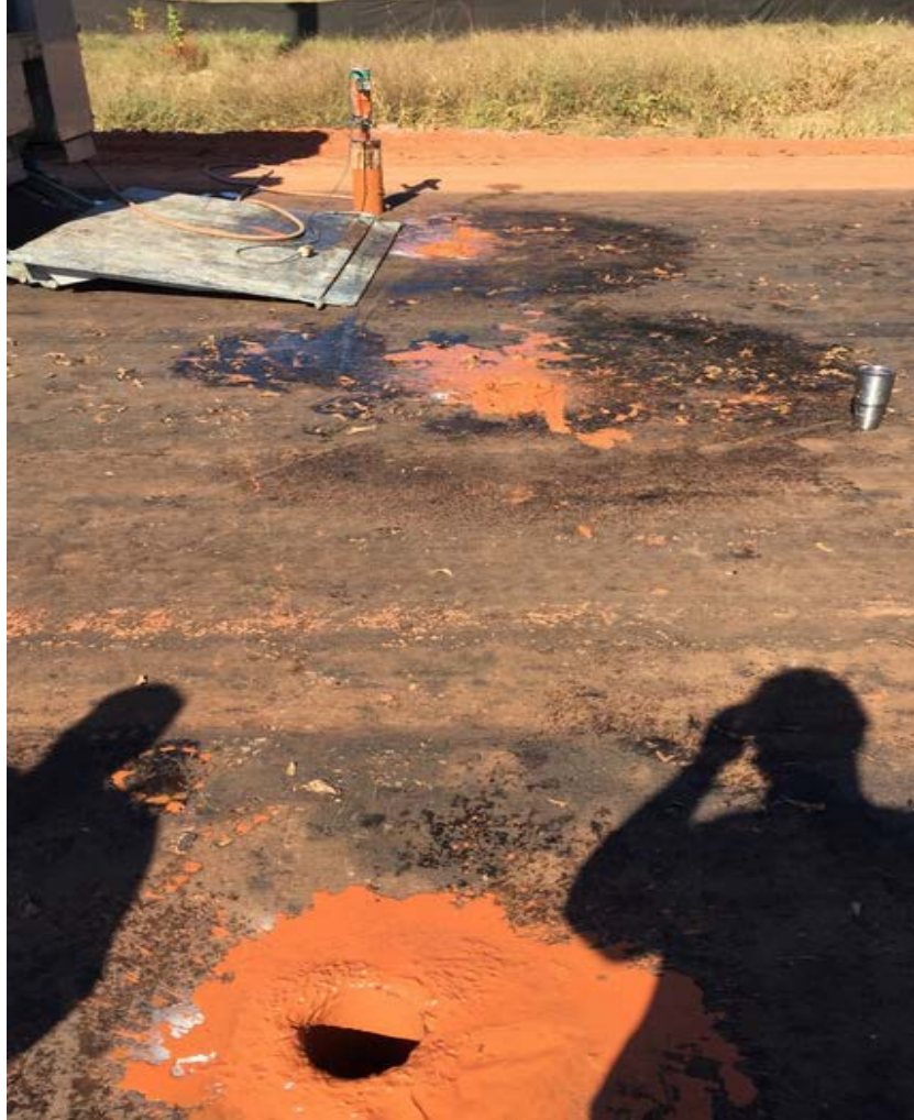
Figure 2.20: Cored section of soil cement ready to be repaired on U.S. Highway 84
