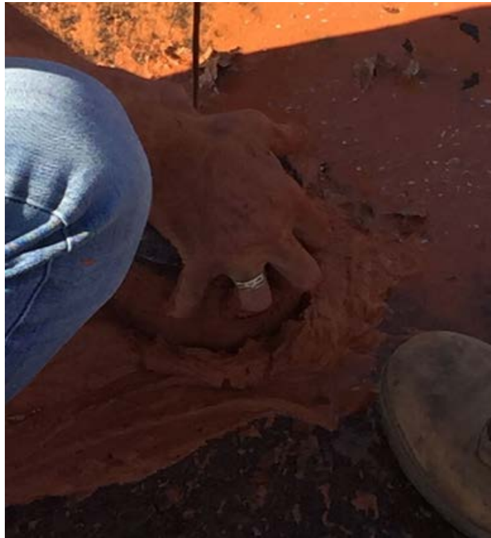
Figure 3.35: Core sample being removed from the soil-cement base on the Elba project
