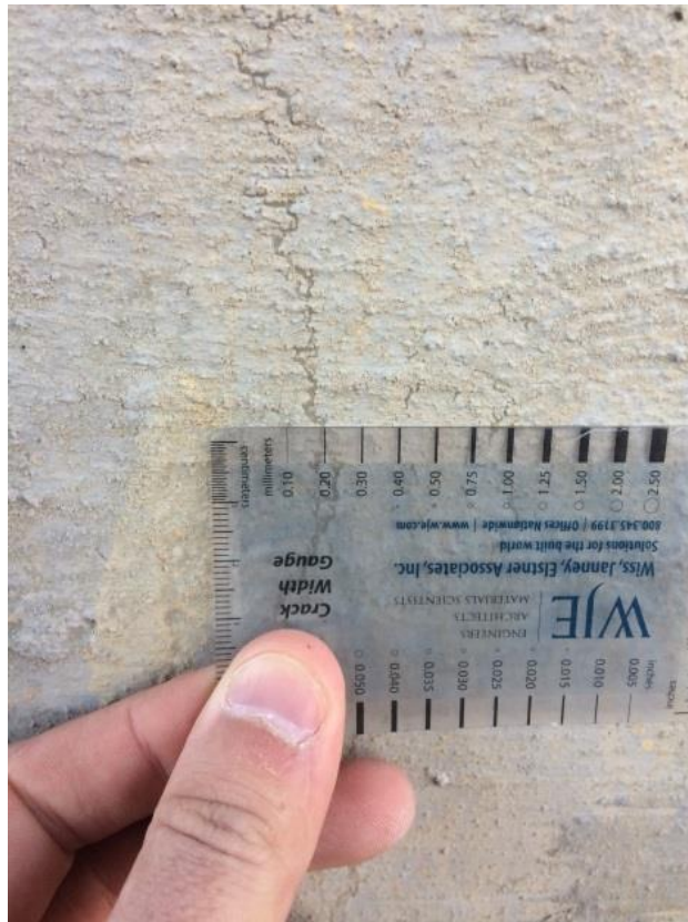
Figure 5-12: Harpersville crashwall crack
