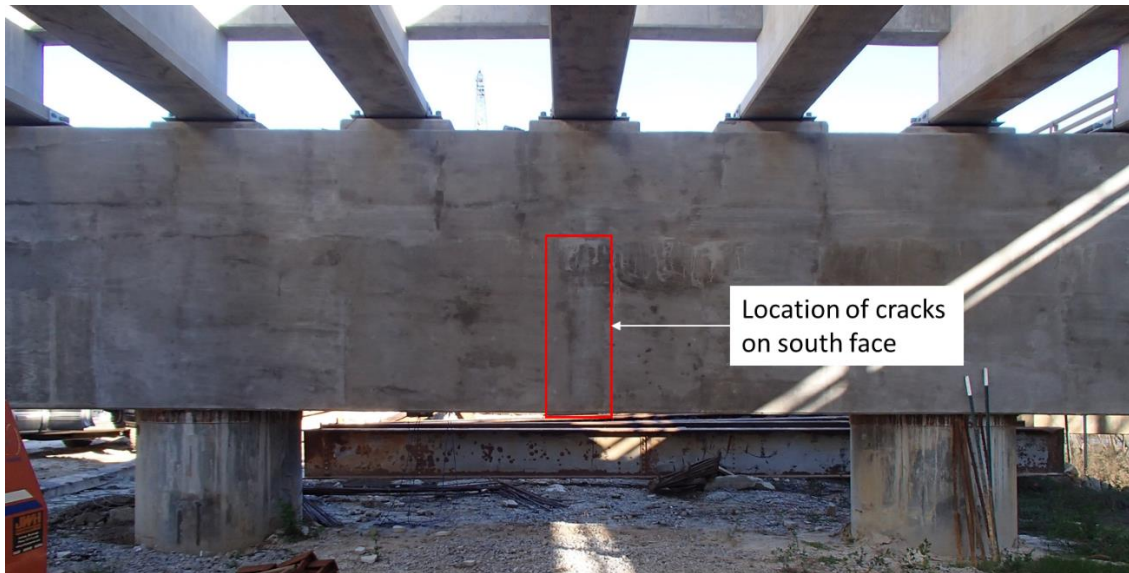
Figure 5-47: Brewton bent cap location of cracks on south face
