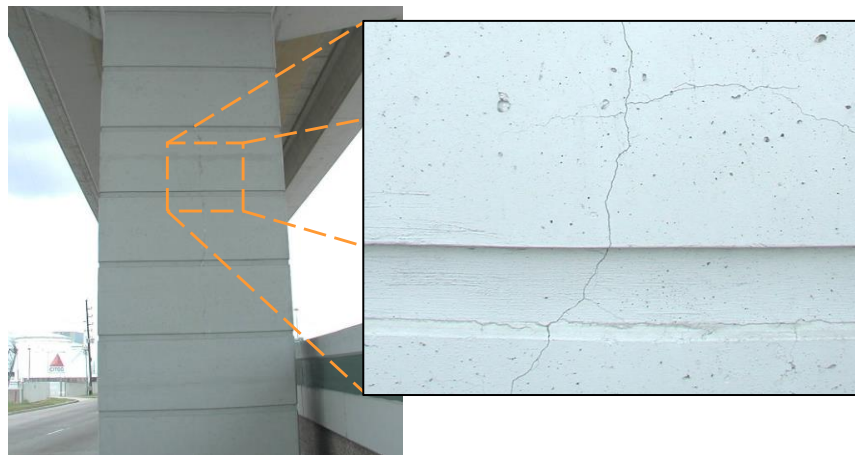
Figure 1-1: Thermal cracking of a bridge column in Texas (Photo Courtesy of Dr. J.C. Liu)
