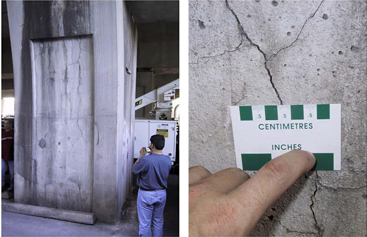
Figure 2-9: DEF induced cracking in San Antonio Y overpass (Thomas et al. 2008)
