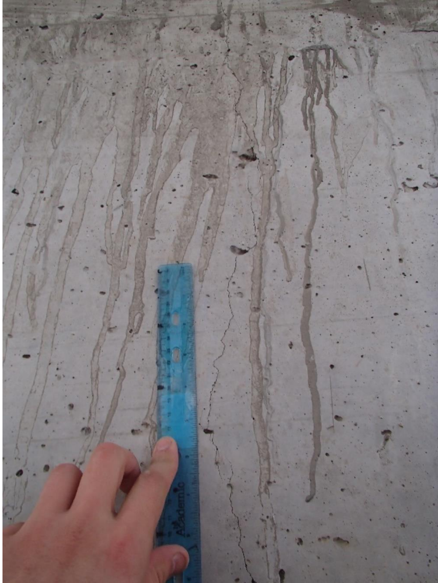
Figure 5-21: Scottsboro pedestal crack 3
