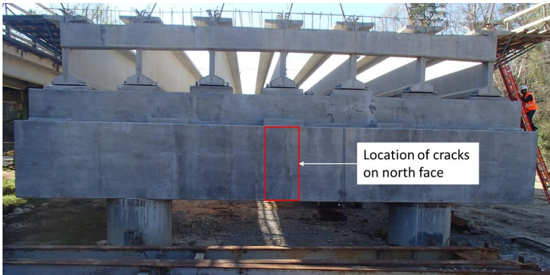
Figure 5-45: Brewton bent cap location of cracks on north face
