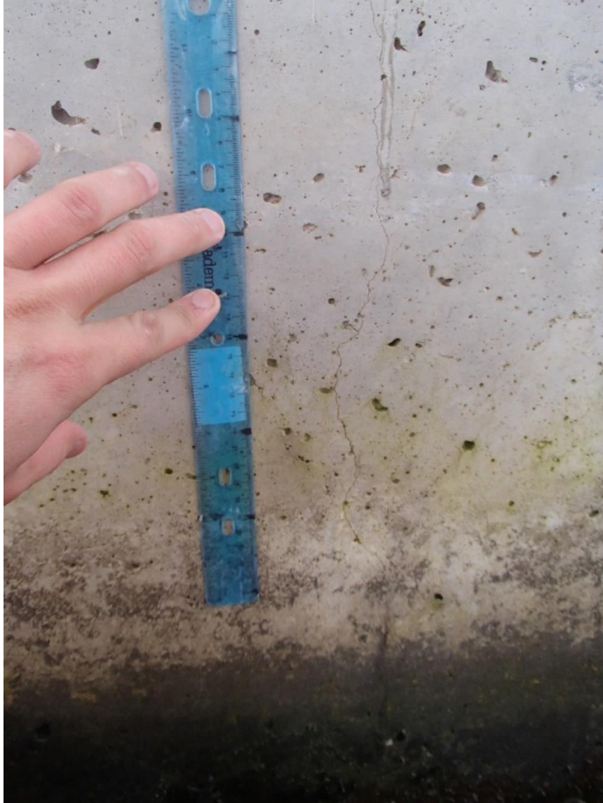
Figure 5-20: Scottsboro pedestal crack 2
