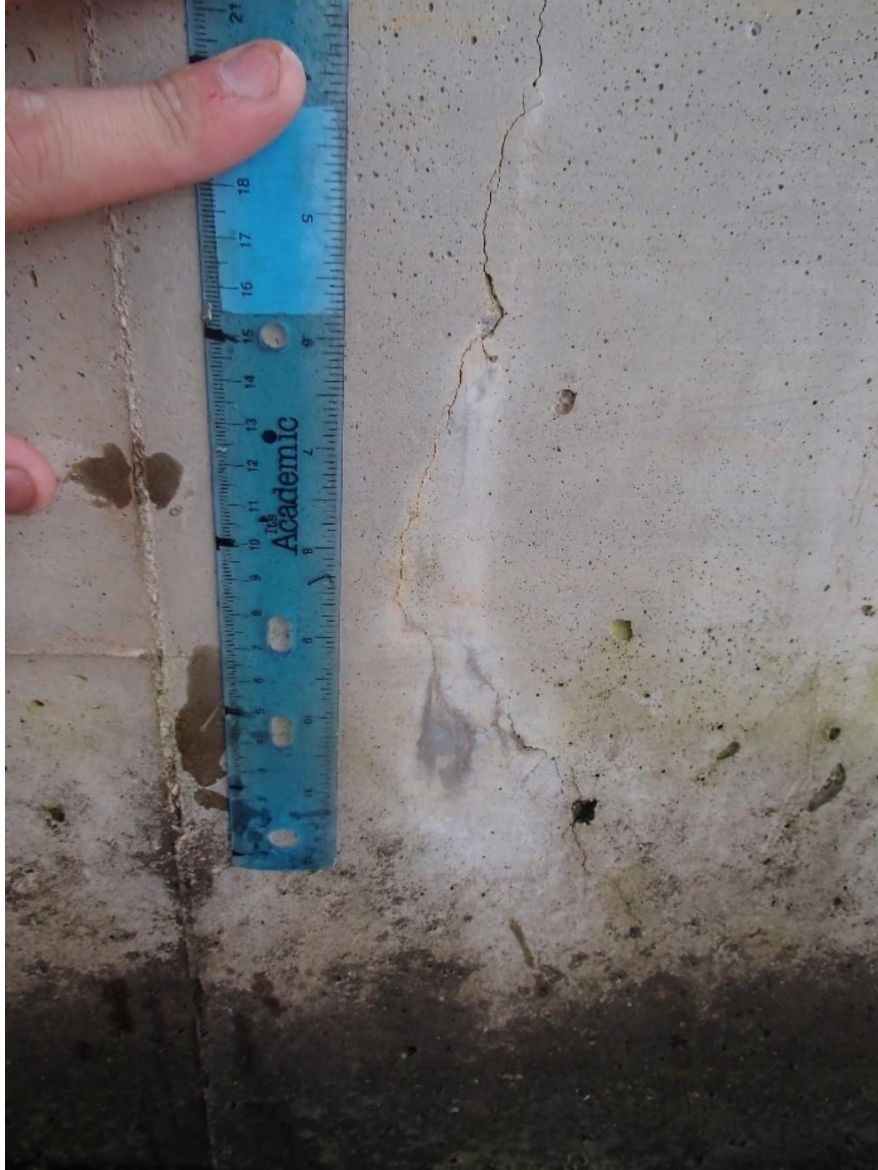
Figure 5-22: Scottsboro pedestal crack 4
