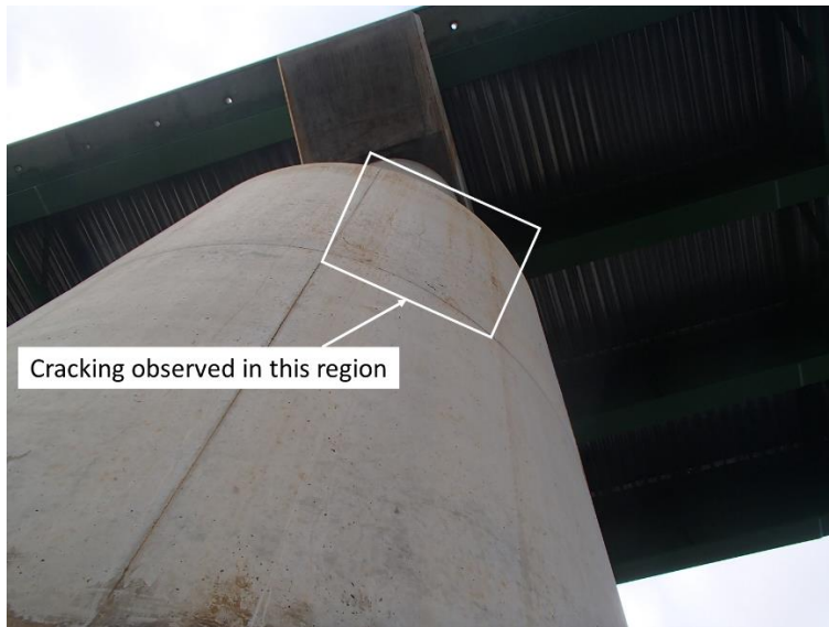
Figure 5-23: Scottsboro pedestal cracks observed at top of pedestal (unreachable)
