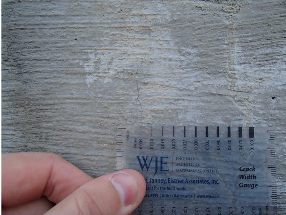
Figure 5-46: Brewton bent cap crack (north face)
