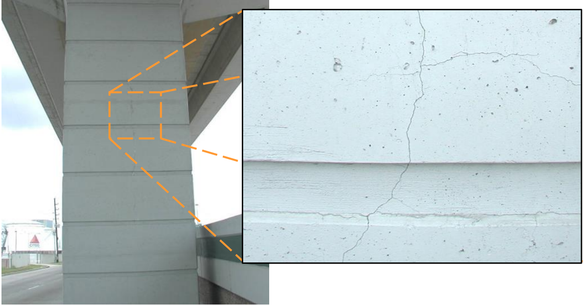
Figure 2-6: Thermal cracking in a Texas bridge element (Photo courtesy of Dr. J.C. Liu)
