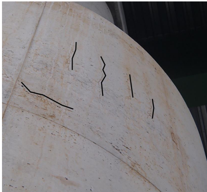
Figure 5-24: Scottsboro pedestal close-up of cracks observed at top of pedestal (unreachable)
