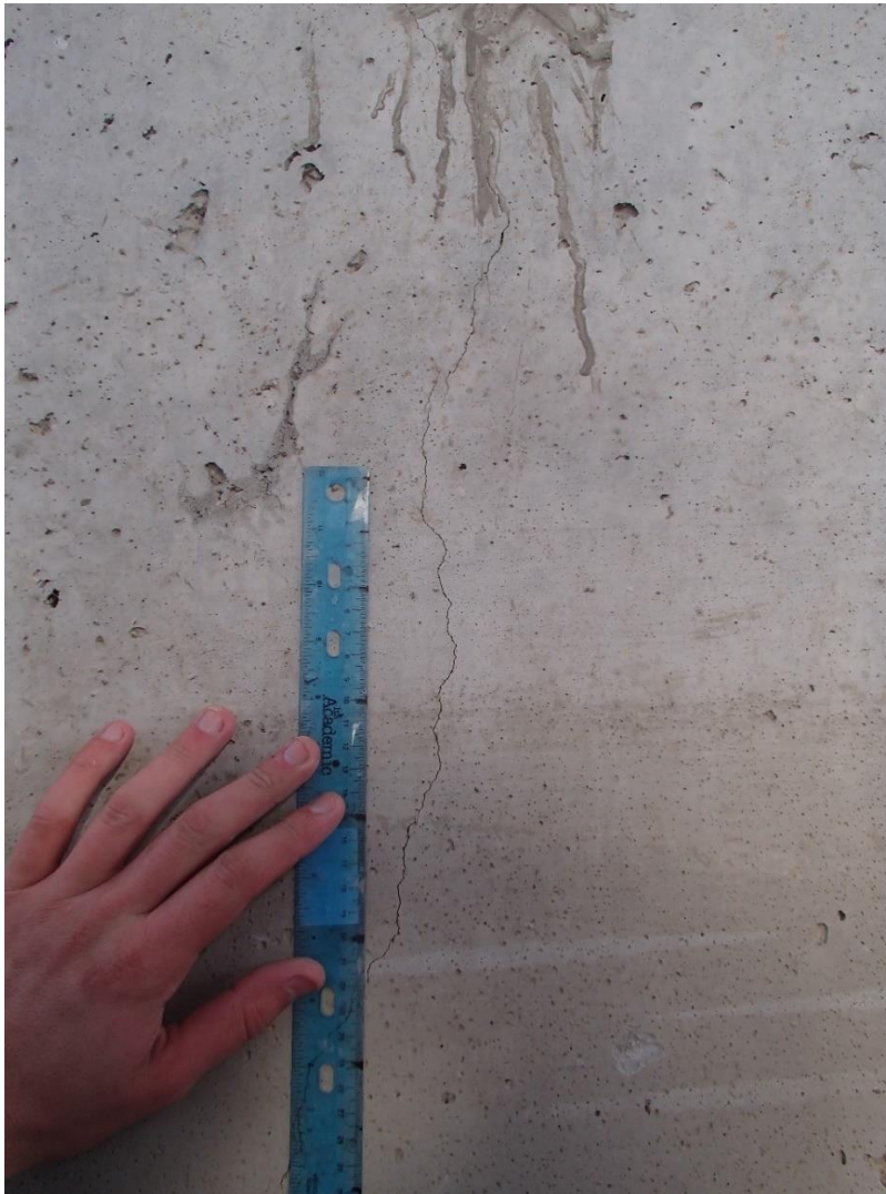
Figure 5-19: Scottsboro pedestal crack 1
