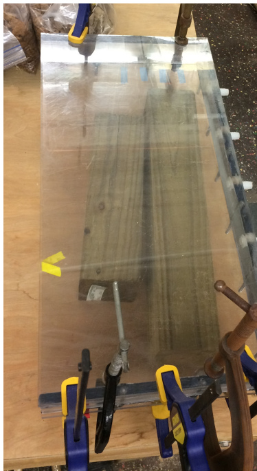
Figure 3.15: Construction of flow cell. Detachable side getting glued together and compressed to allow the epoxy to set. Used acrylic sheets with dimensions of 62.5 x 5 x 32.5 cm (24.6 x 2 x 12.8 in) and glued together with epoxy (Gorilla Epoxy, The Gorilla Glue Company, Cincinnati, OH, USA) and sealant (LEXEL Elastic Sealant, Sashco, Inc., Brighton, CO, USA).
