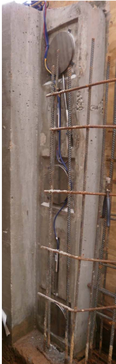
Figure 4-2: Post installed pressure cells
