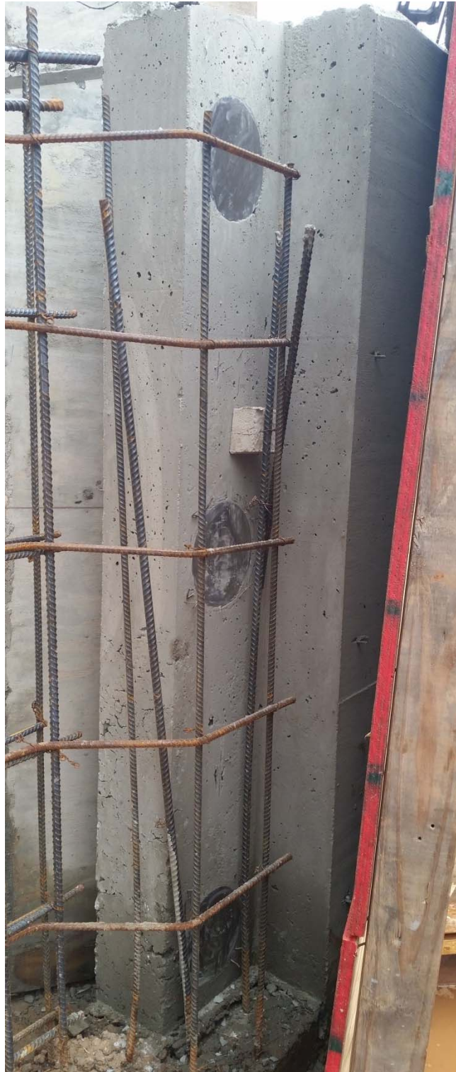
Figure 4-4: Pressure cells embedded in culvert tab
