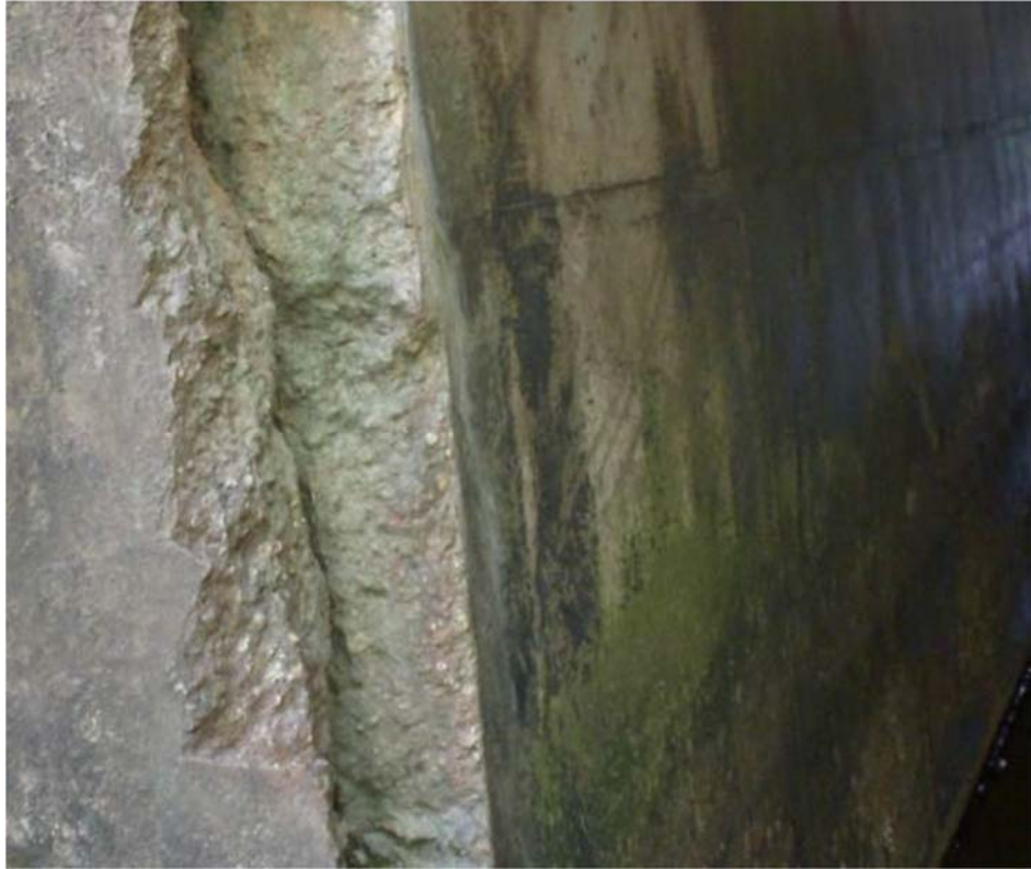
Figure 1-1: Distress at Wing Wall Connection to Culvert (Minton, 2012)
