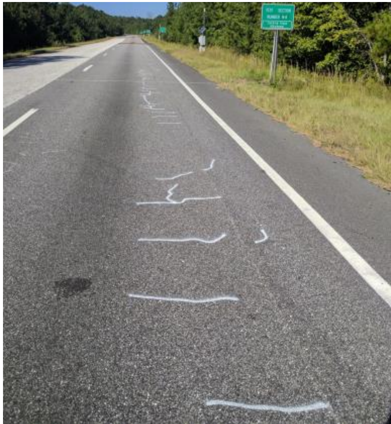
Figure 29. Mapped cracks on Test Track section
