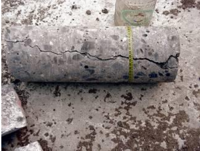
Figure 8-2: Cored concrete from footing when the insulation blew off during cold weather conditions (Courtesy: CTL Group)
