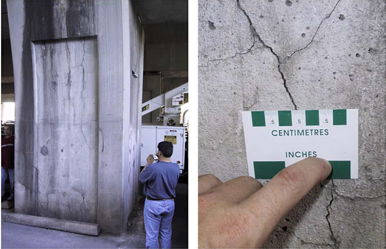
Figure 2-3: Cracking due to DEF at the San Antonio Y overpass (Thomas et al. 2008)
