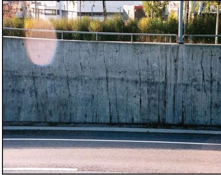
Figure 9-3: Thermal cracking in concrete barrier walls (Bjontegaard 2013)
