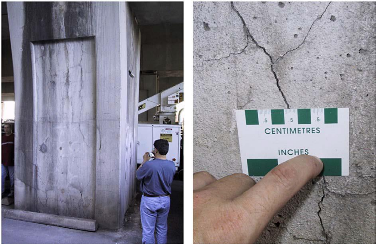
Figure 1-3: Cracking due to DEF at the San Antonio Y overpass (Thomas et al. 2008)
