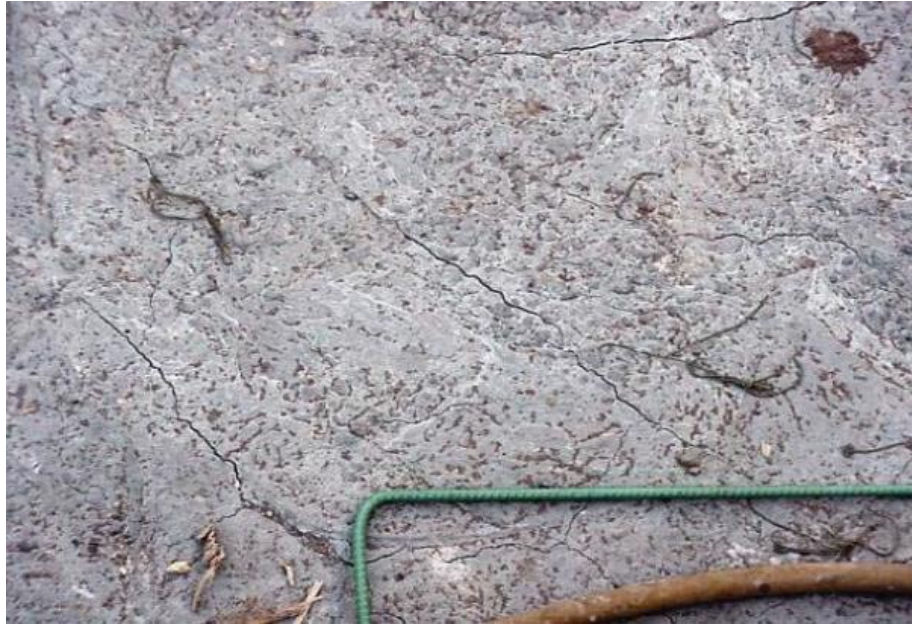
Figure 3-4: Thermal cracking observed in a thick slab (Gajda 2007)
