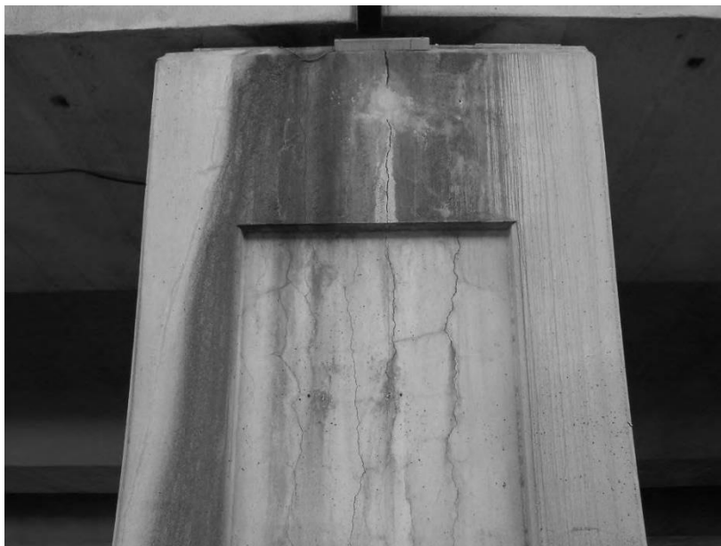
Figure 3-3: Cracking observed in a mass concrete column due to DEF (Folliard et al. 2006)
