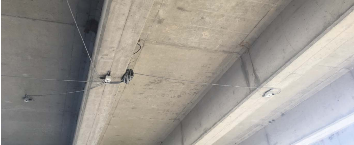
Figure 0-2. Placement of SiWIM Strain Transducers - Bridge Weigh-in-Motion
