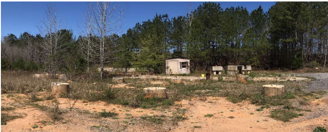
Figure 15. Photo of drilled shafts looking from south to north taken in March 2018.
