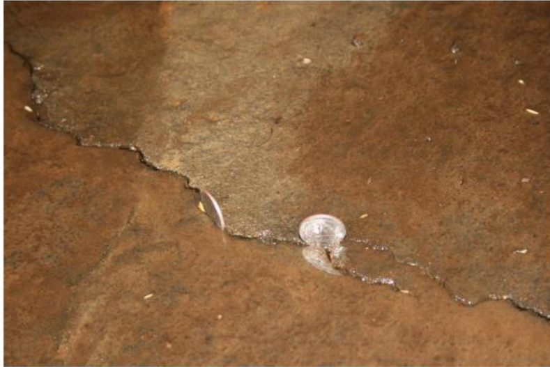
Figure 10-2 Transverse base crack in the AEB project (crack width>0.06 in.) (Minton 2012)
