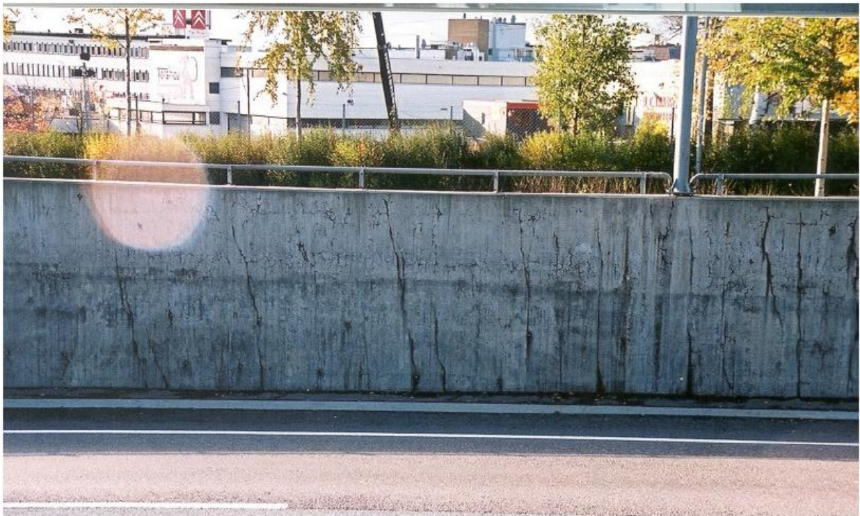
Figure 1-2 Thermal cracking in walls due to external restraint provided by footing
