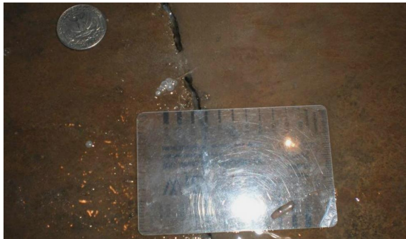
Figure 10-11 Base Crack from AEB Culvert at 240+37 (Minton 2012)
