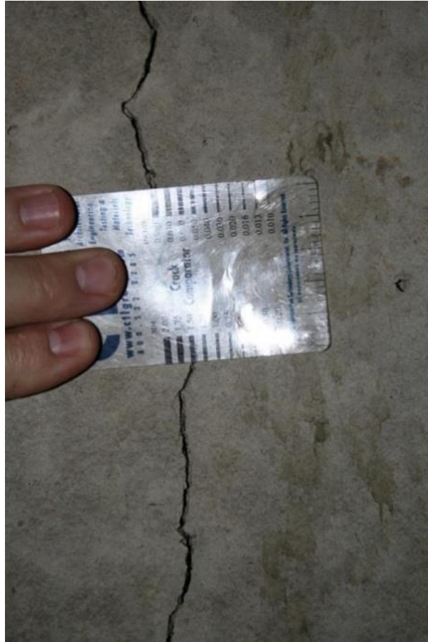
Figure 9-1 Cracking in culvert wall
