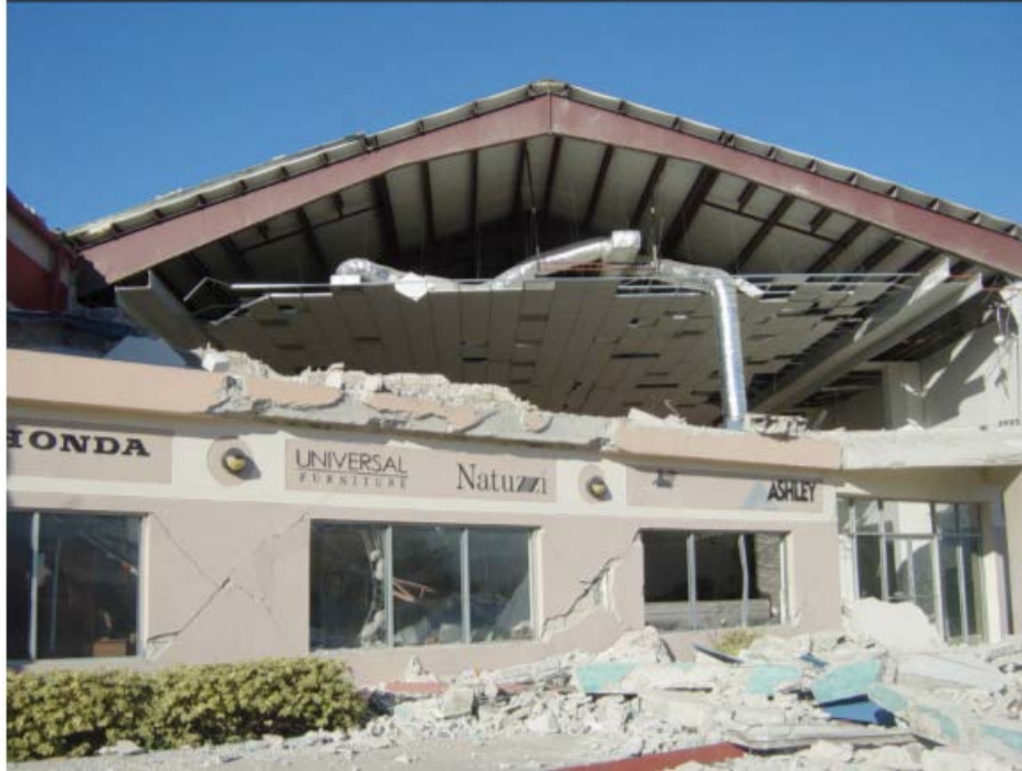
Figure 2-22. Infill Masonry Wall Collapse of PEMB in Port-au-Prince (Eberhard et al. 2010)
