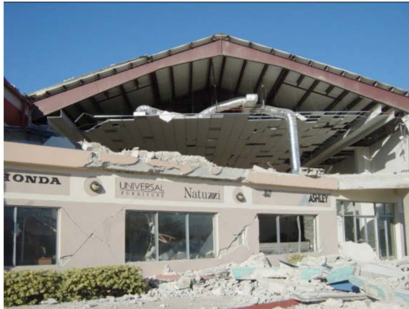
Figure 1-2. Infill Masonry Wall Collapse of PEMB in Port-au-Prince, Haiti (Eberhard et al. 2010)
