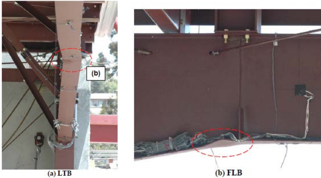
Figure 2-14. Buckling around the Pinch Point (Smith 2013b)
