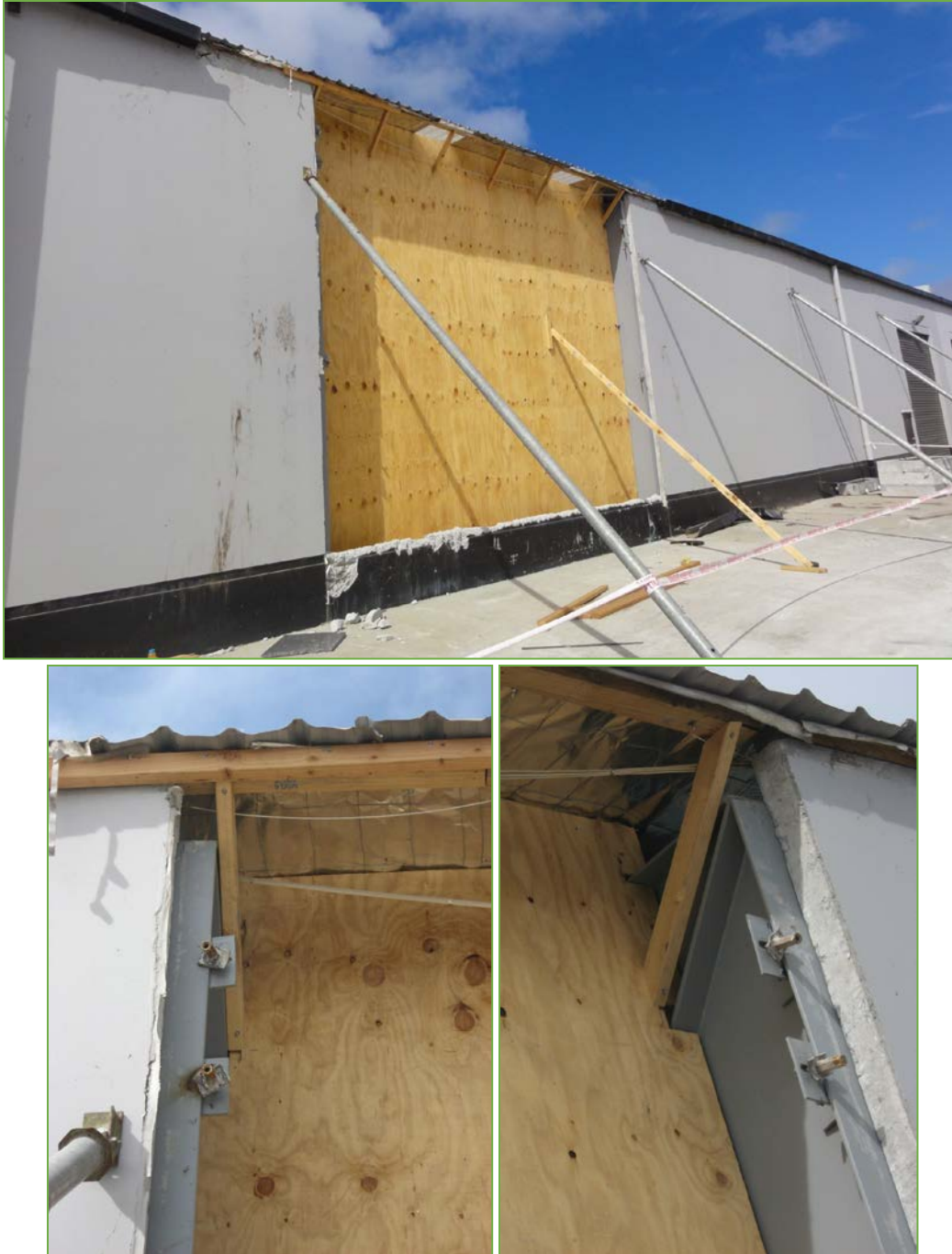
Figure 1-1. Loss of panel and temporary shoring of adjacent panel in Christchurch, New Zealand (Marshall and Gould 2012)
