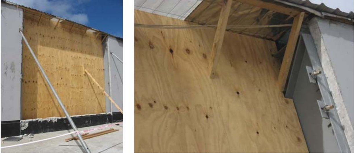
Figure 2-23. Loss of panel and temporary shoring of adjacent panel (Marshall and Gould 2012)
