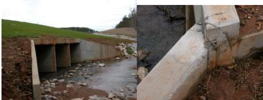
Figure 1-1. Culvert distress on AL 49 near Dadeville, AL
