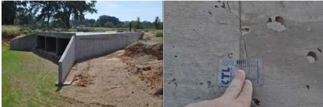
Figure 1-2. Culvert distress near Centerville, AL
