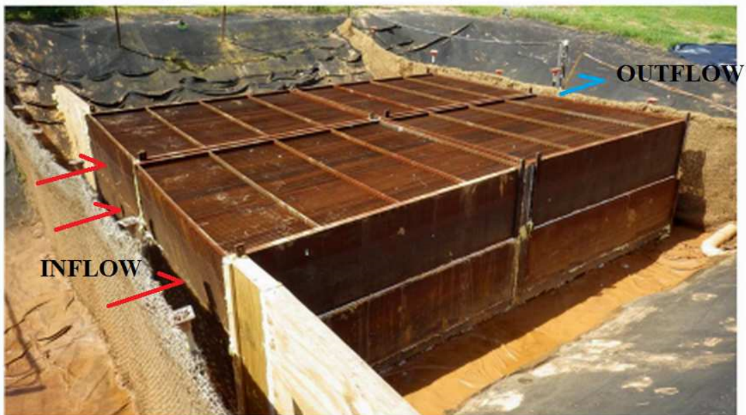
(b) Sediment basin - Configuration 4
