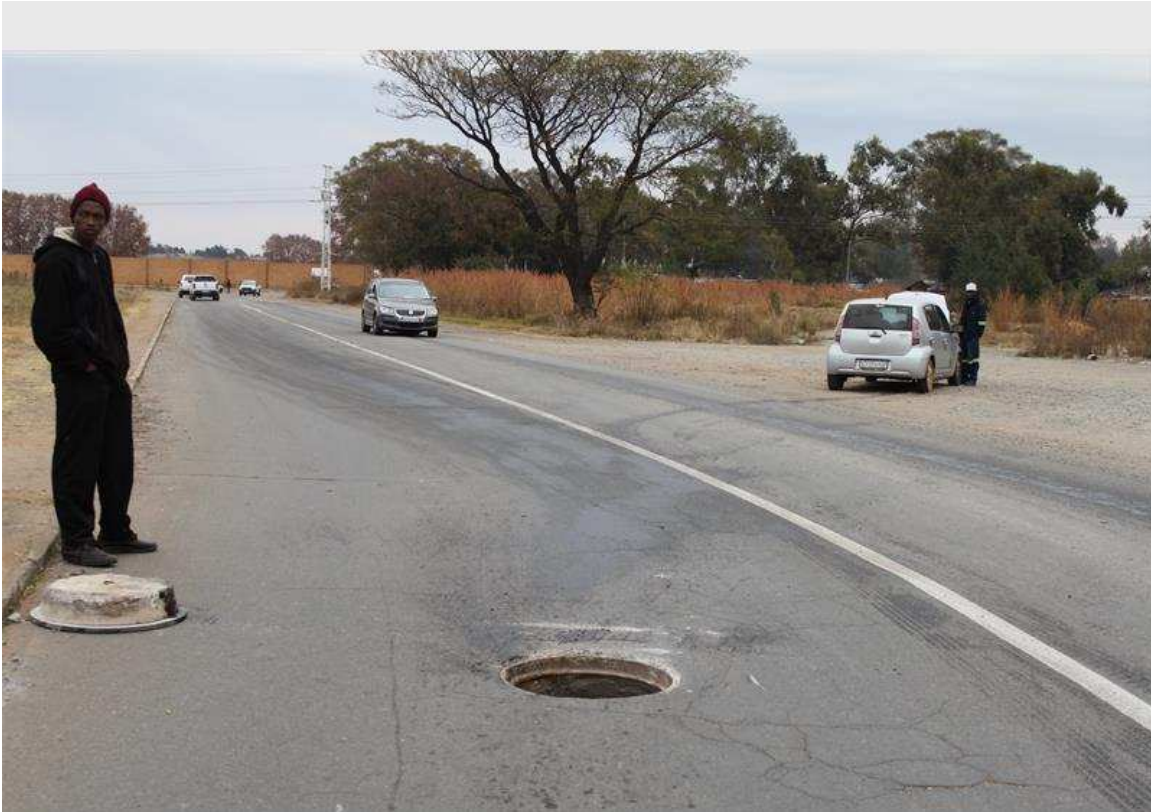
Figure 2.4: Example of a displaced manhole cover causing a traffic accident (Fourie, 2015).
