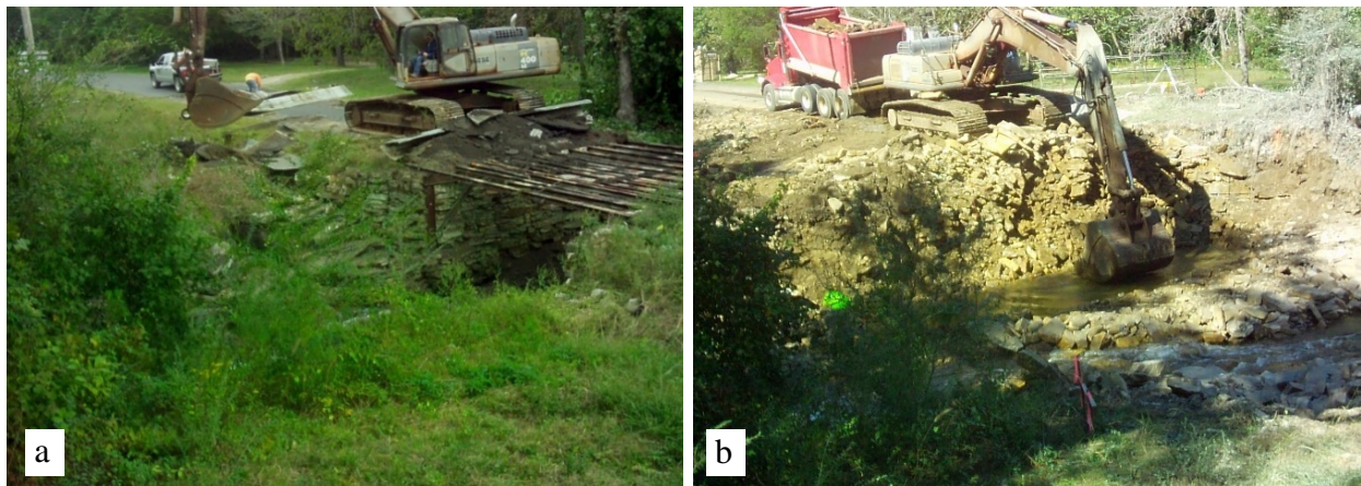
Figure 20: (a) Removal of the existing bridge at Turkey Creek; (b) removal of blasted sandstone, on the western side of Turkey Creek.
