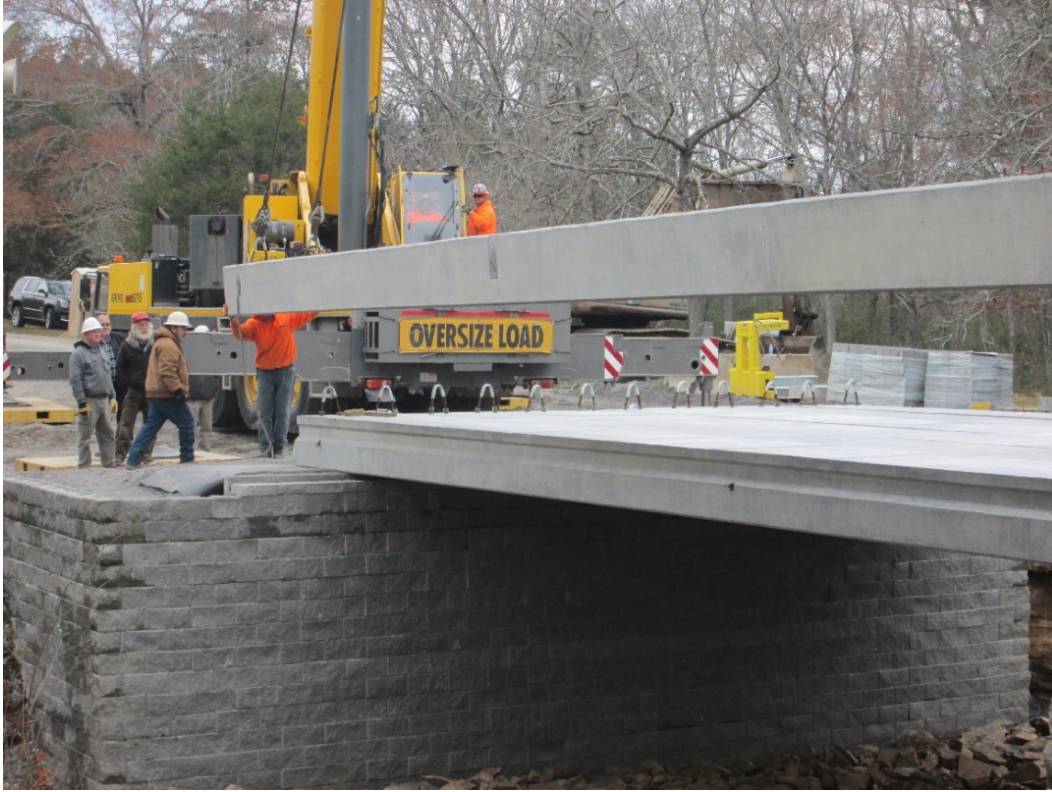
Figure 2: Placing prestressed concrete box beams onto the beam seat of the Marshall County GRS with segmental retaining wall (SRW) unit facing.
