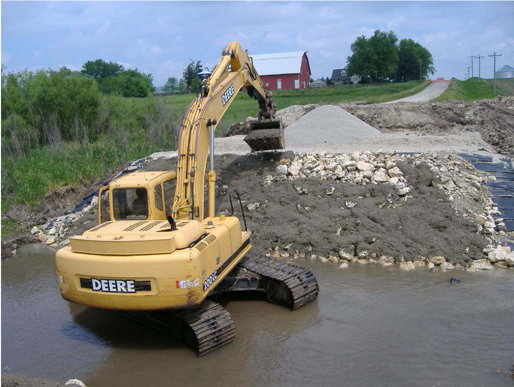
Figure 1: Olympic Avenue GRS abutment in Buchanan County, Iowa. Abutments use grouted riprap over wrapped geosynthetic face for scour protection (photo from Vennapusa et al. 2012).
