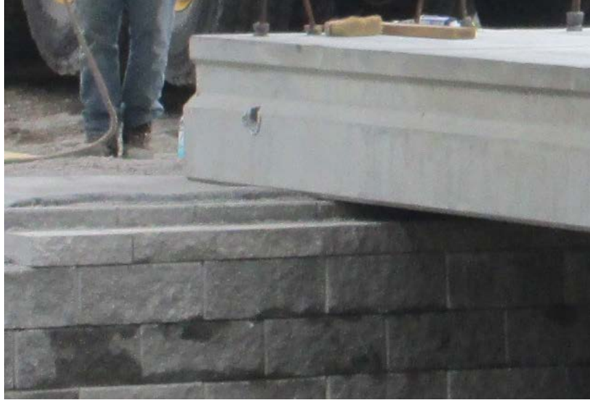
Figure 24: Bridge beam setting on top of CMU with 3 in. gap between abutment and beam and integrated approach reinforcement layer. The circular opening for post-tensioning can be seen at the end of the beam.
