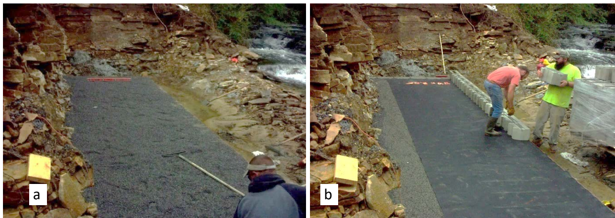
Figure 22: (a) Placement of initial layer of No. 89 stone to top of first row of masonry blocks and (b) placement of geosynthetic and second row of masonry blocks.
