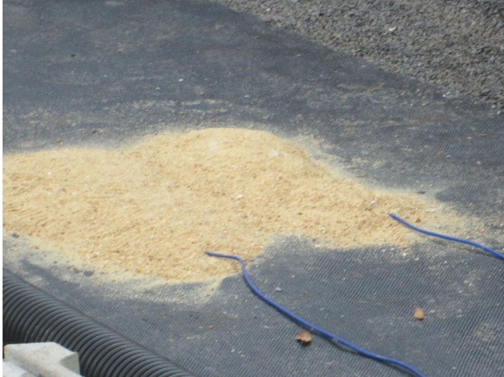
Figure 33: Installed earth and pore pressure sensors covered with sand to mitigate arching
