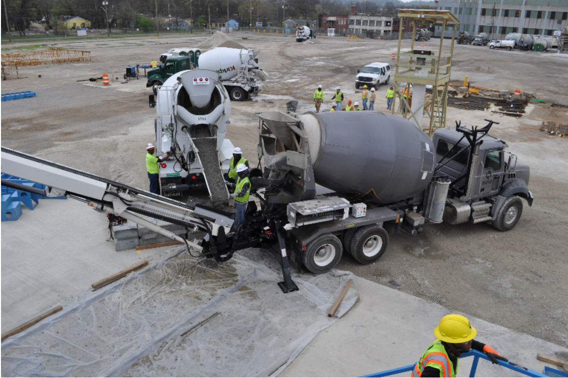
Figure 4-8: Concrete being discharged onto to belt conveyor for transport to the segment
