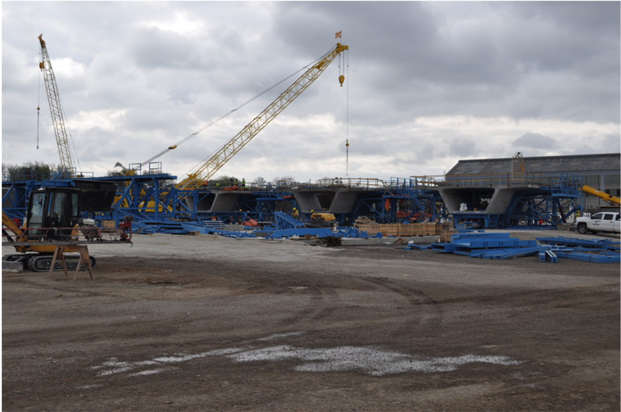
Figure 1-2: Concrete segments and formwork used in the construction of the I-59/I-20 segmental bridge replacement
