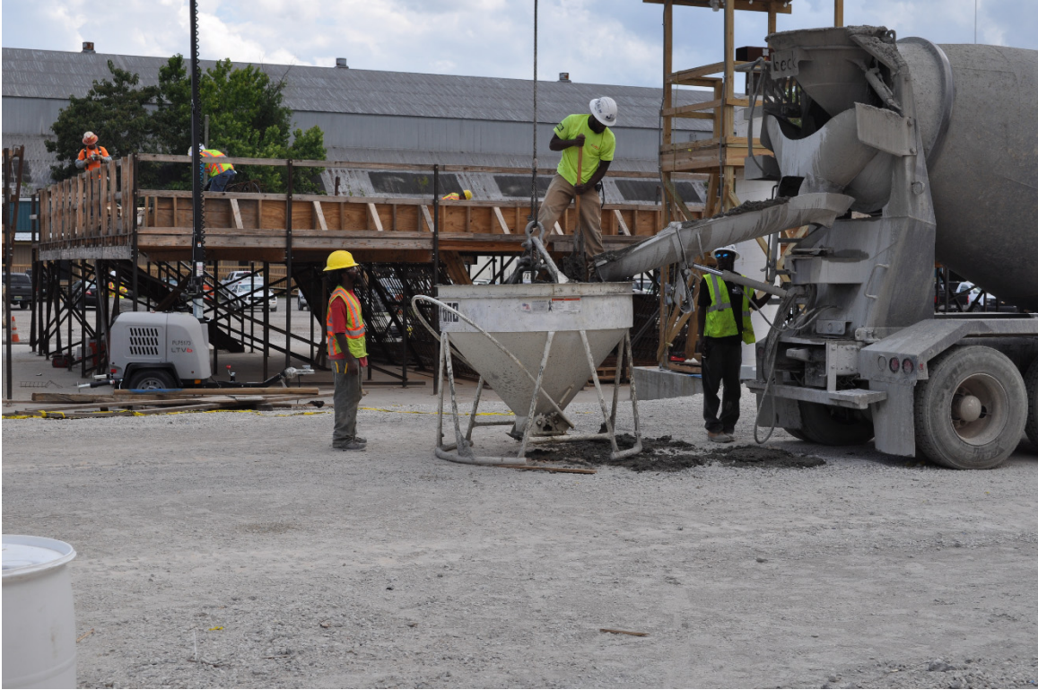
Figure 4-9: Concrete being discharged into a concrete bucket for transport to the segment
