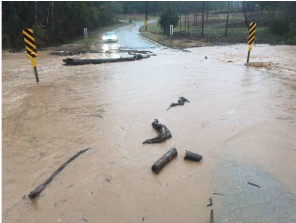
Figure 1.3: Overtopping at Dean Road Bridge during a storm event of 02/03/2016
