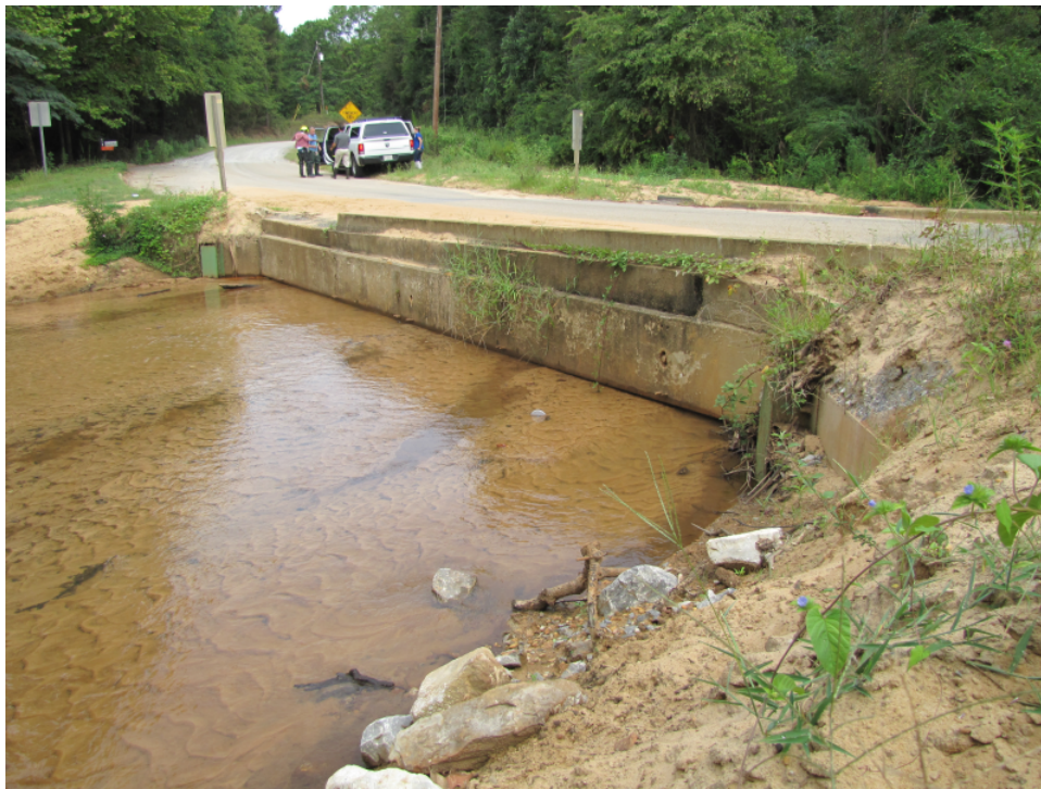
Figure 1.2: Aggradation in Soapstone Branch under Dean Road Bridge (Field visit on 8/11/2015)
