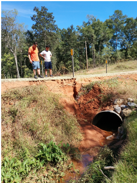
Figure 5.27: Surface erosion in the eastern embankment and erosion created by stormwater flows from Dean Road, creating slope failures immediately upstream from the temporary steel bridge.
