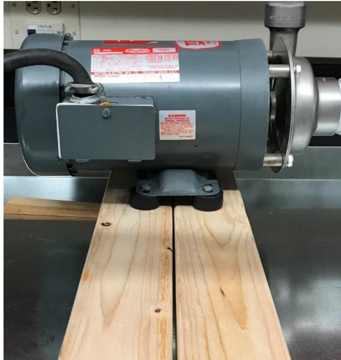
Figure 5.2. Pump resting on rubber spacers and mounted on wood blocks
