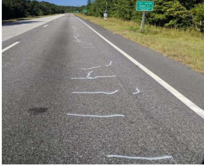
Figure 23. Crack Mapping on the Test Track (Giler, 2017)
