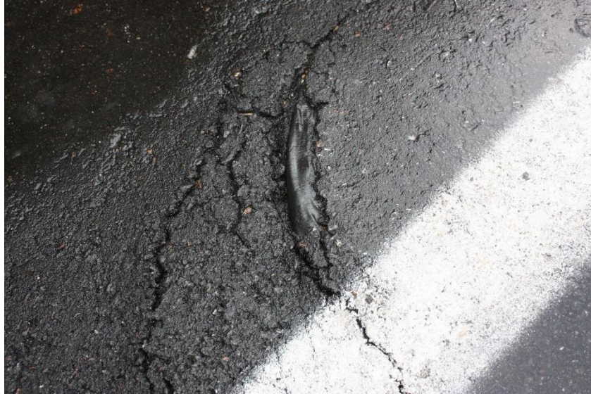
Figure 32: Geosynthetic Protruding Through Base Course of Asphalt
