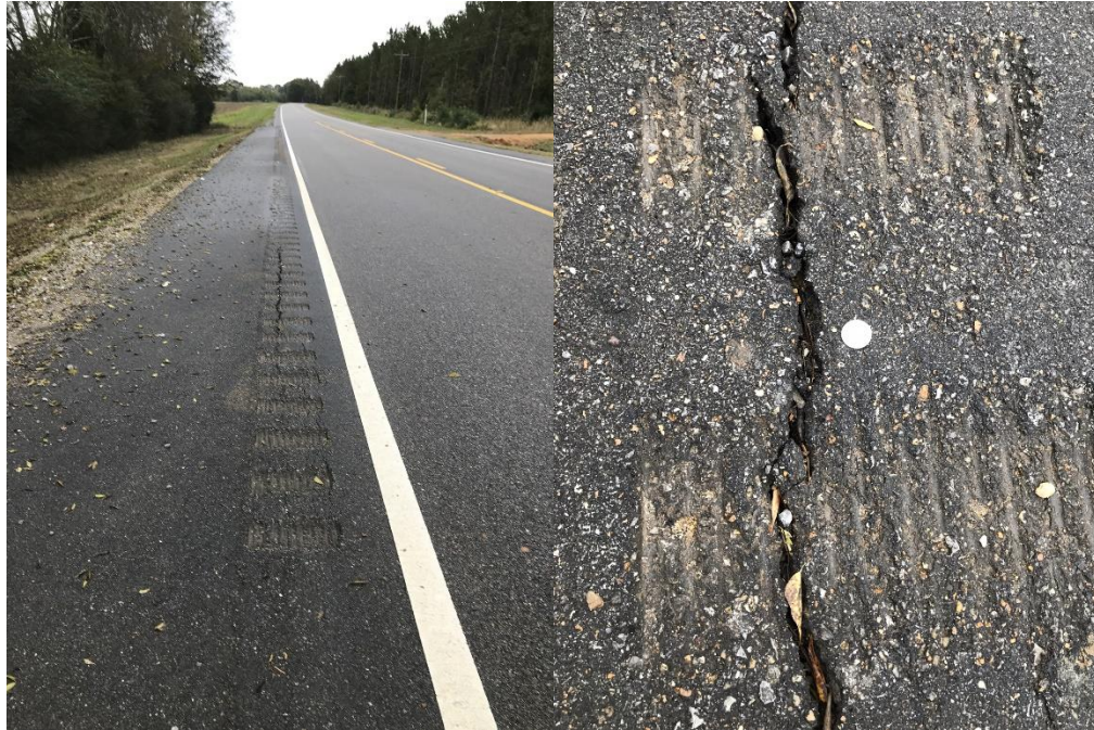
Figure 109: Cracks in Paved Shoulder Test Section November 2018
