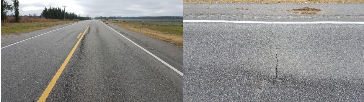
Figure 111: Pavement Distress and Cracks in Paved Shoulder Test Section December 2018
