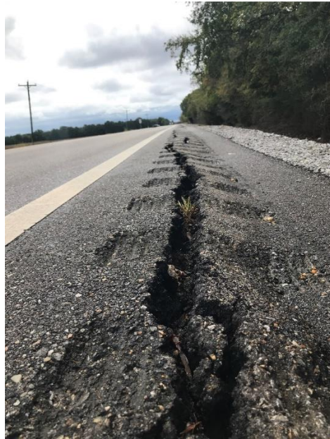
Figure 113: Vertical Barriers Crack October 2019
