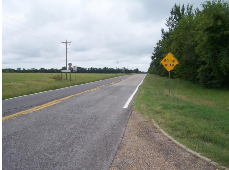
Figure 1: Distress Pavement at AL-5 (Herman 2015)
