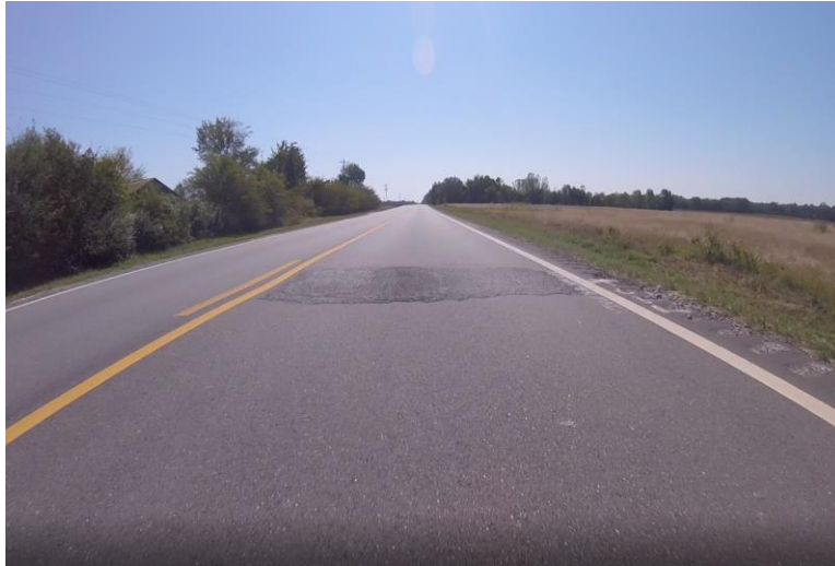
Figure 105: Location of IRI Spike (Culvert Patch) in Southbound Lime Columns Section September 2017
