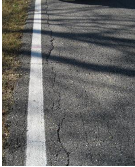
Figure 38: Longitudinal Crack Along Edge of AL-5
