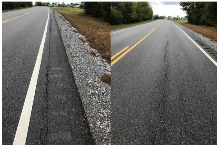
Figure 114: Shoulder and Lane Cracking in the Edge Drain Test Section October 2019
