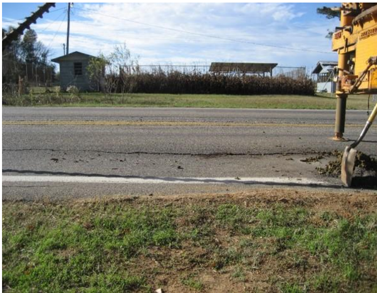
Figure 2: Longitudinal Cracking along AL-5 (Herman 2015)
