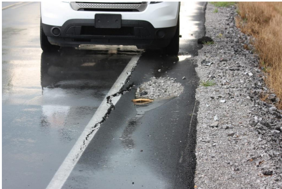
Figure 31: Cracking and Rutting Observed above Vertical Barriers
