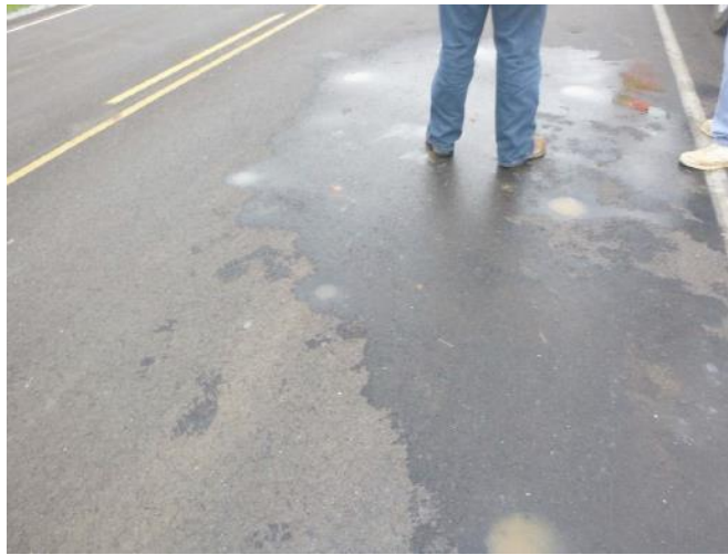
Figure 37: Lime Columns Reflected Through Base Course and Holding Water
