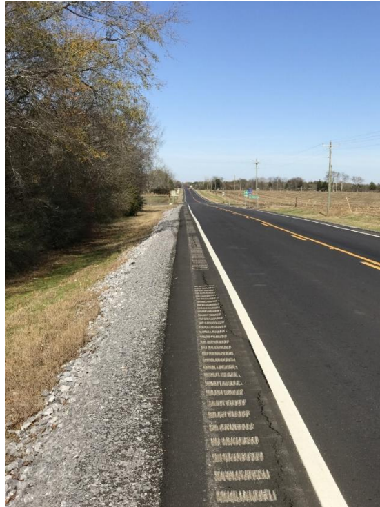
Figure 104: Longitudinal Crack in Vertical Barrier Section December 2016
