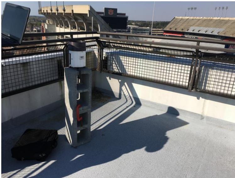
Figure 2.10: Rain Gauge Installed on Top of Haley Center
