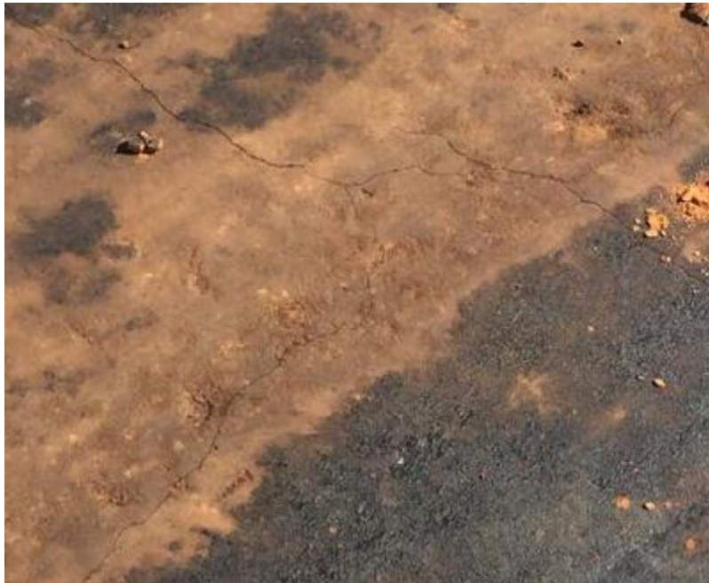
Figure 2.8: Shrinkage cracks in soil cement (McLaughlin 2017)
