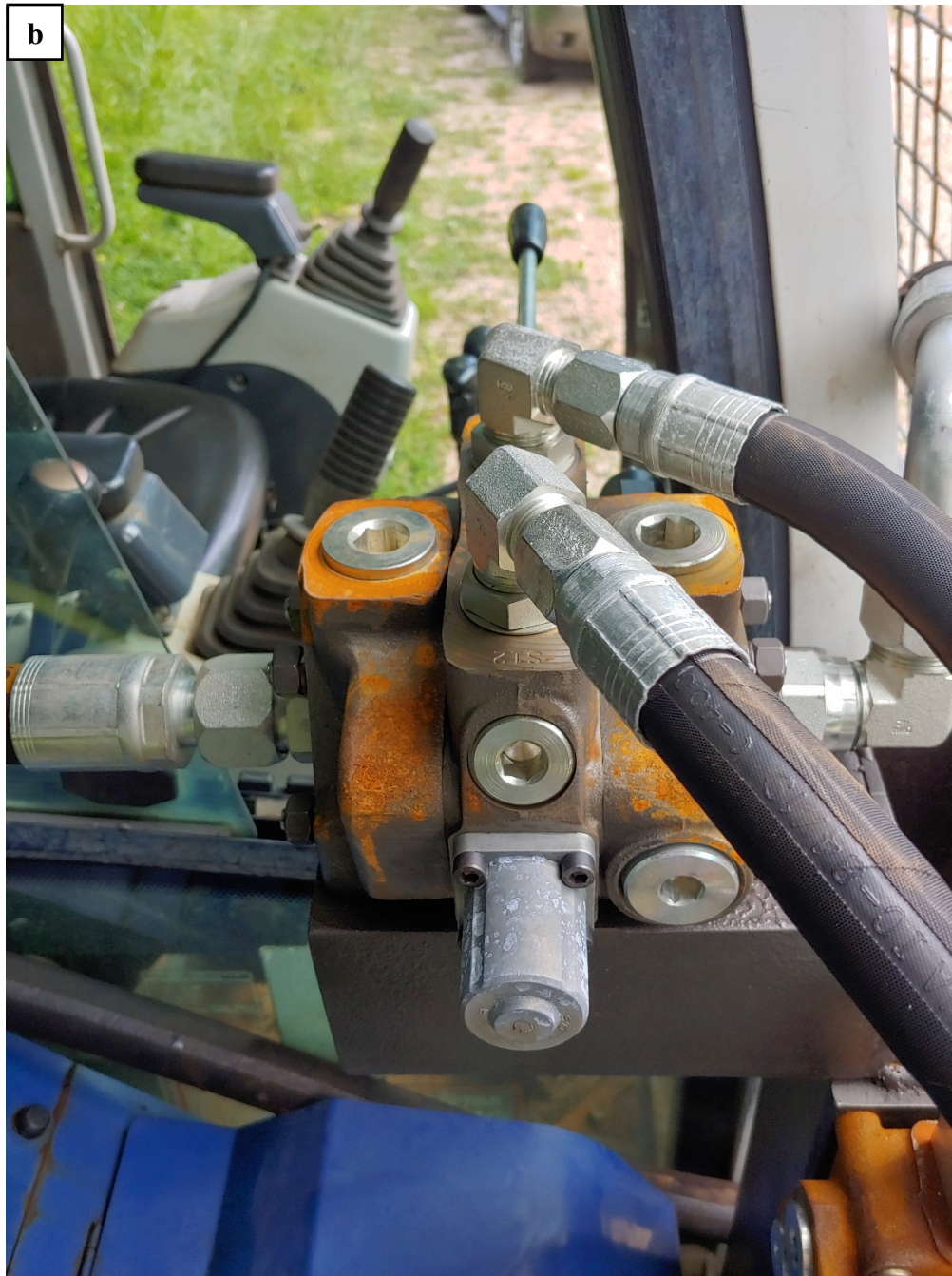
Figure 14. Hydraulic hoses connected to the actuator responsible for opening and closing of the shear.
