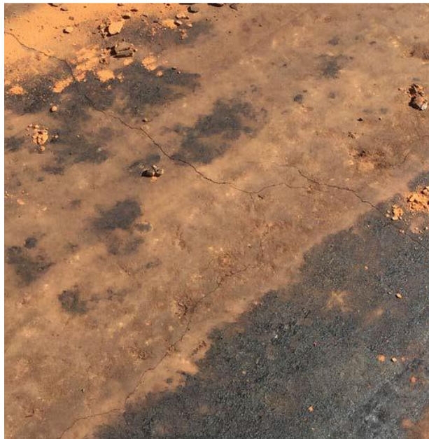
Figure 0.7: Transverse and longitudinal cracking on U.S. Highway 84 (McLaughlin 2017)
