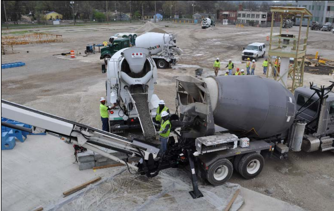
Figure 4-8: Conveyor moving concrete to desired location at the top of the formwork
