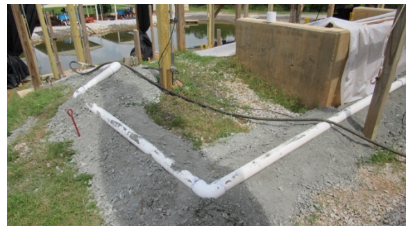
(b) 3-inch (7.62 cm) distribution system
