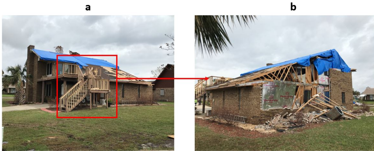
Figure 3.17: Another example on anchoring the sides of the structure based on details in structure or the surroundings. a) the left side of the structure, which was impacted by Hurricane Michael (2018), has an outdoor staircase which is indicated by the red square. b) a small part of the staircase can be seen where the red arrow is pointing. This indicates that this is of the back of the structure.
