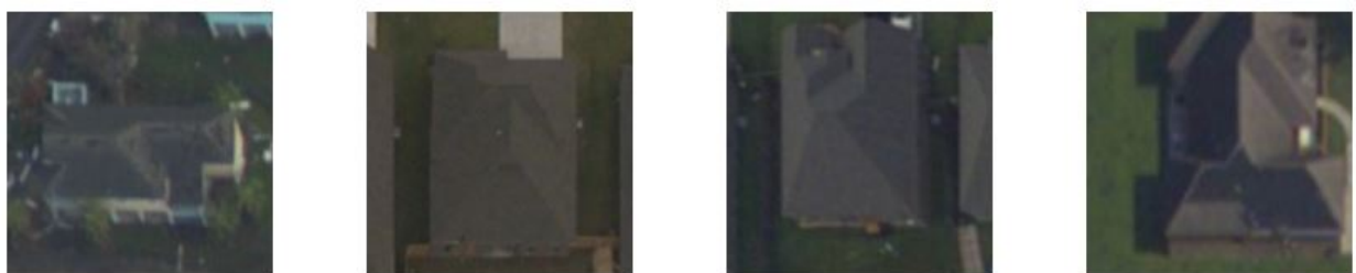
Figure 4.11: Roofs that were classified as undamaged but based on StEER's data are labeled as minor damage. These images show how easy it is to misclassify minor and undamaged roofs using aerial imagery only.
