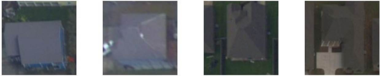
Figure 4.12: Roofs that were classified as minor but based on StEER’s data are labeled as undamaged. These images show how easy it is to misclassify minor and undamaged roofs using aerial imagery only.
