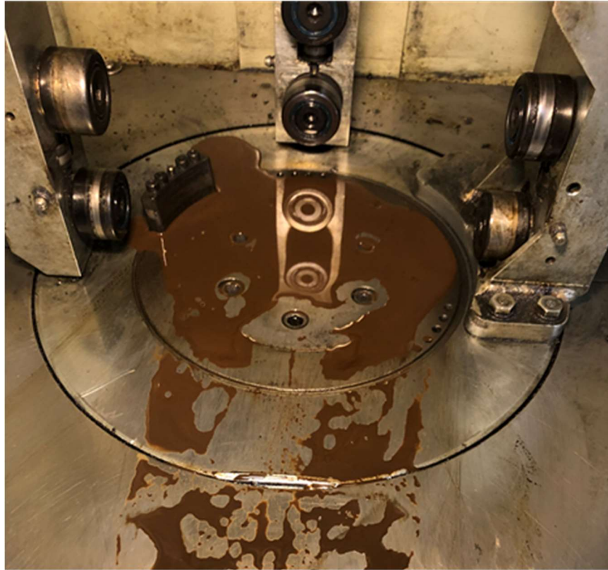
Figure 58: Engineered Emulsion and water seepage from compacting the 5.4% moisture content as-built CCPR-E mixture.
