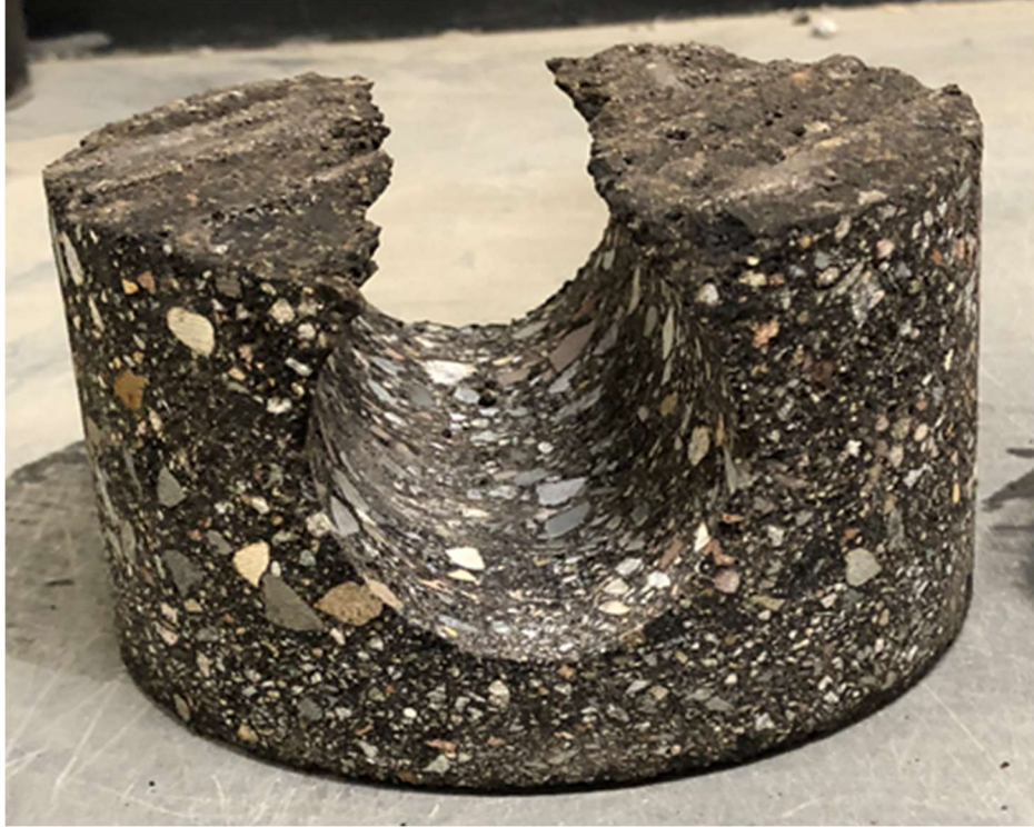
Figure 35: Cold recycled field core sample with the milled pavement surface exposed as a result of too thin a lift.
